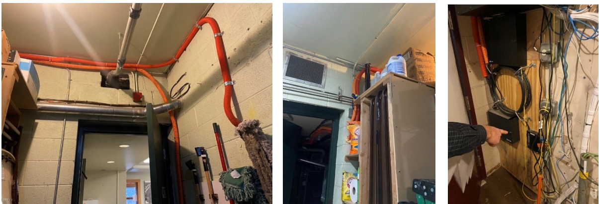
Figure 5 Fiber Optic Cable and Splice
