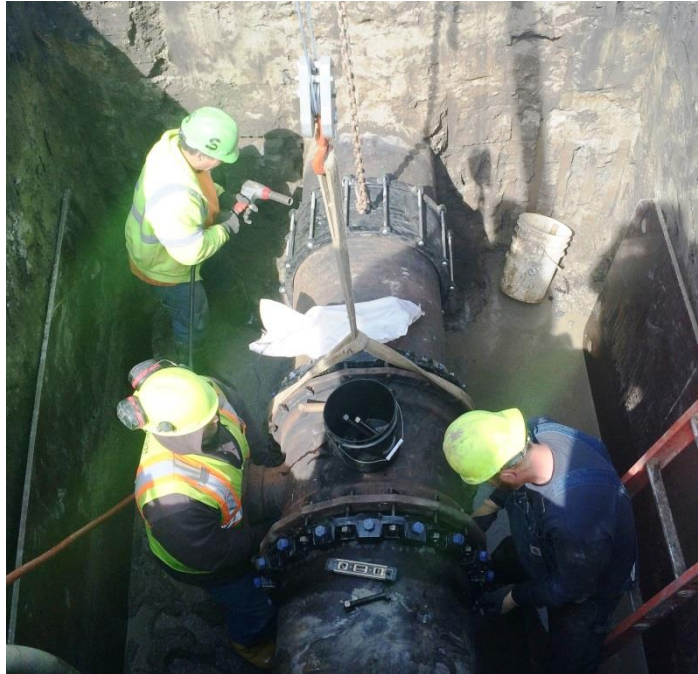
A Distribution Division field crew installing a new fire hydrant connection on a 24" diameter water main, to improve the City's ability to clean and test this main.
