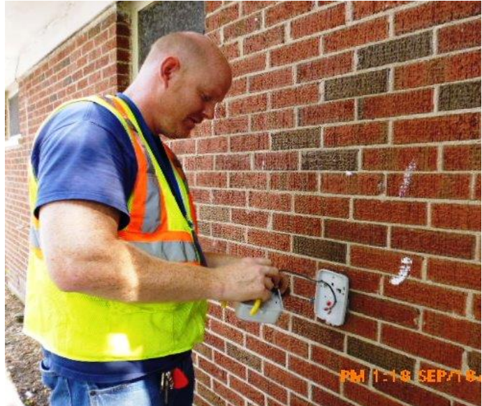
A Public Works Agency employee installs a new remote water meter reading unit on the exterior of a home as part of the Advanced Metering Infrastructure (AMI) software. This unit makes it possible for meter readings to be transmitted via wireless network without City staff having to visit each property to manually read the meters.
