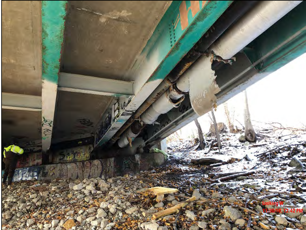
Photo 9: Deck underside configuration West Span. Failed pipe insulation in north bay.
