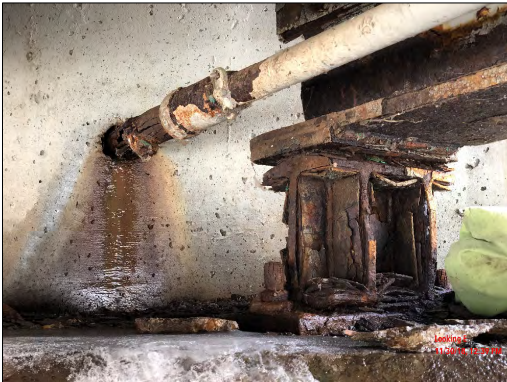
Photo 10: Looking at North abutment bearing. Typical abutment bearings condition at both abutments, with heavy corrosion.
