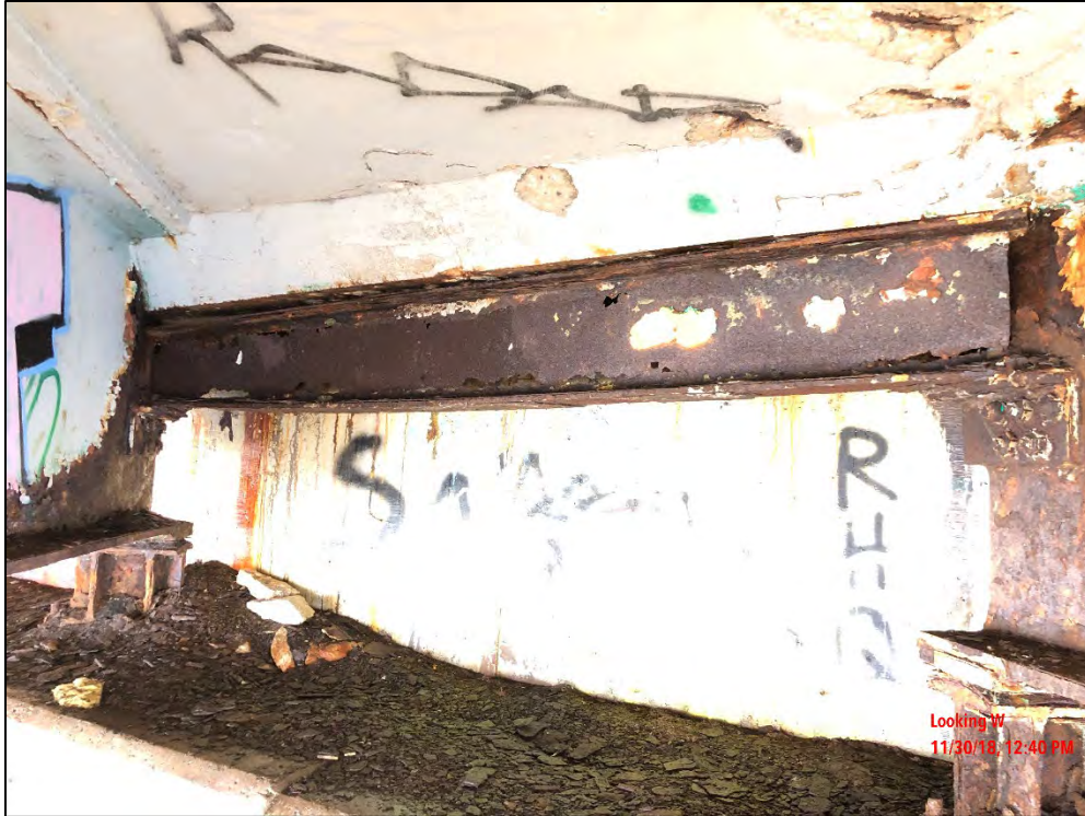
Photo 11: Full section loss of the diaphragm web. Looking at the second diaphragm from the north end at the west abutment.
