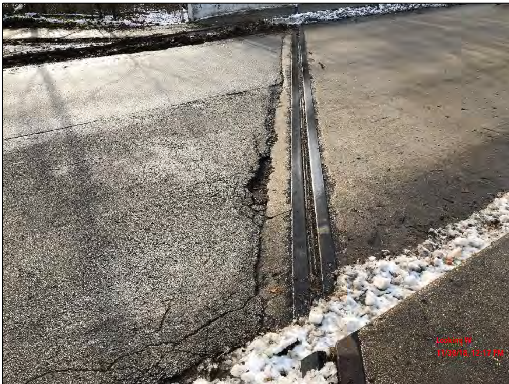
Photo 2: Noted spalled HMA area and map cracks at the east approach.
