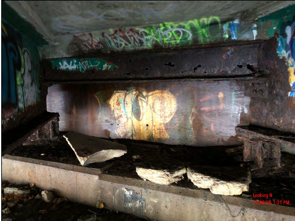
Photo 17: East abutment diaphragm in 2 nd bay from south end of bridge with complete section loss of the web noted at several locations.
