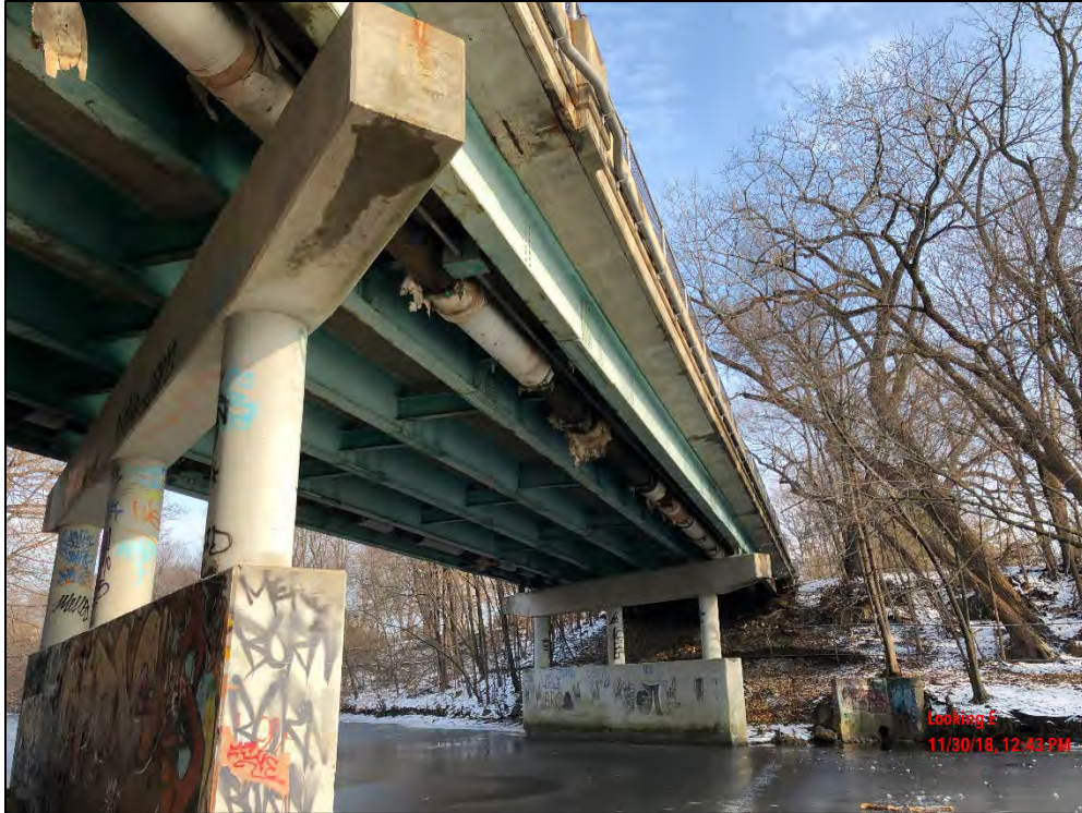
Photo 15: Overall underside of center span. Utility insulations have failed.
