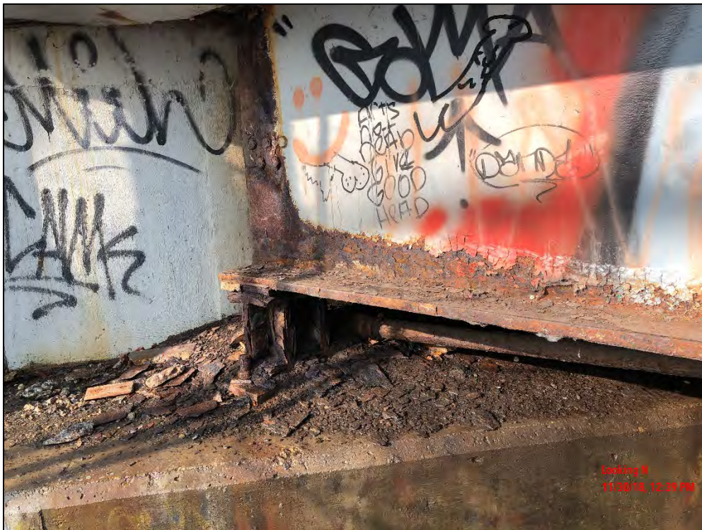
Photo 14: Section loss at south fascia beam and bearing at West abutment.
