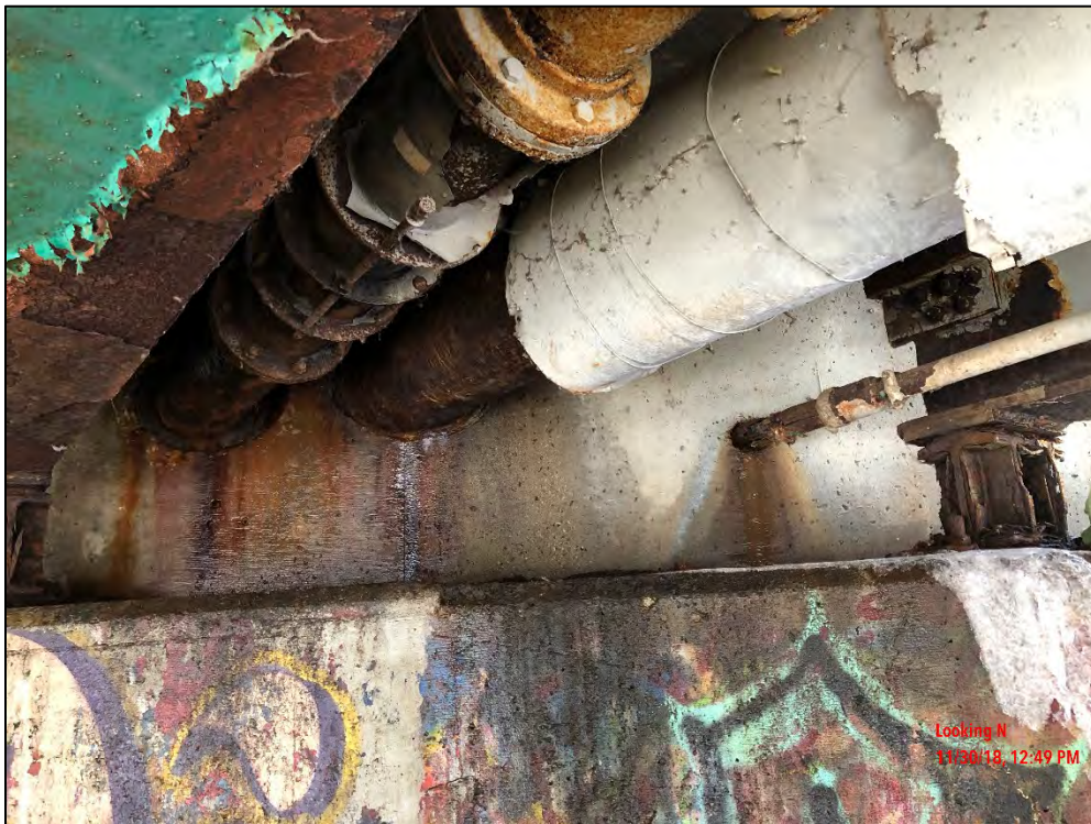
Photo 20: Backwall noted with water seepage at the connection with utilities. Typical condition for both abutments.
