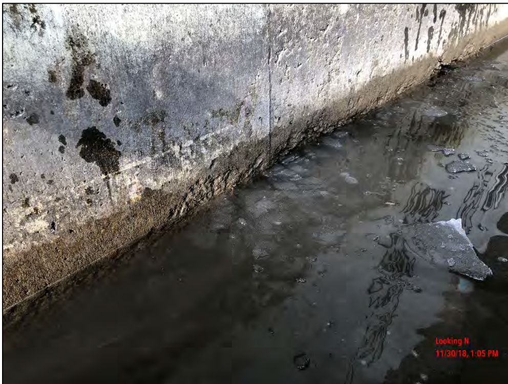
Photo 24: Spalled area, south of photo 23, noted measuring 5' height x 1' depth.
