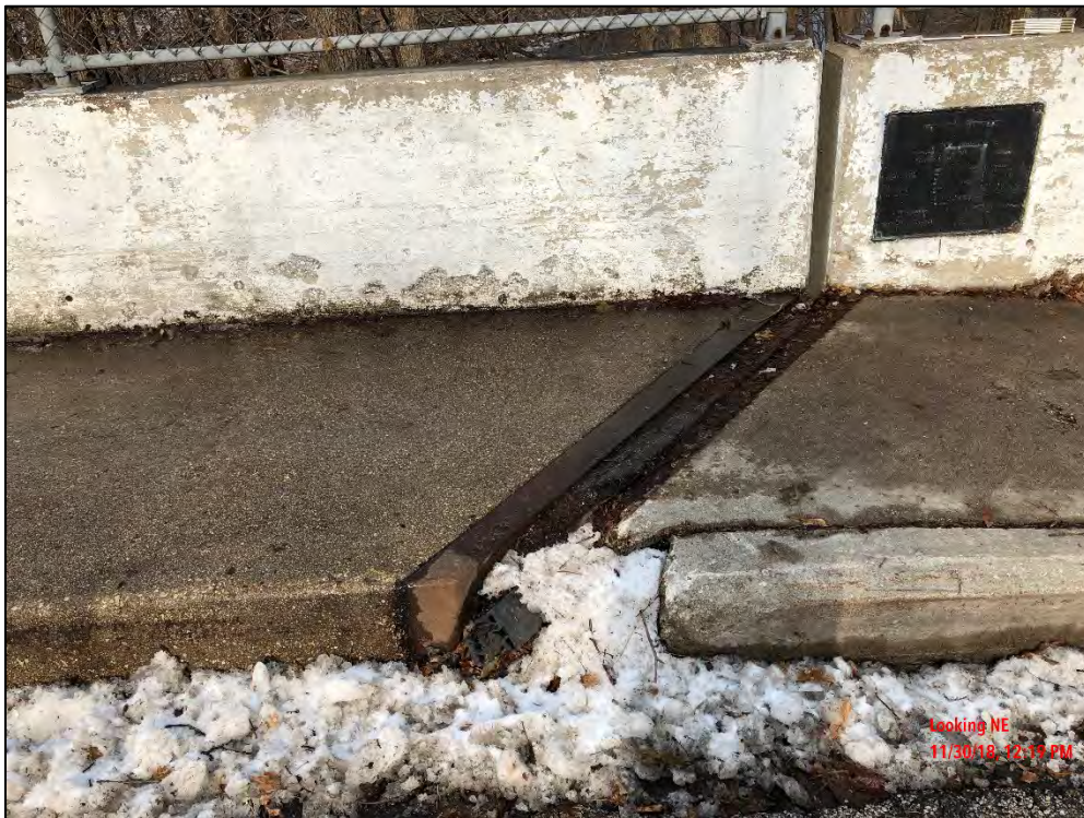
Photo 8: Noted localized spalled area with failed expansion joint gland at north end of the sidewalk.
