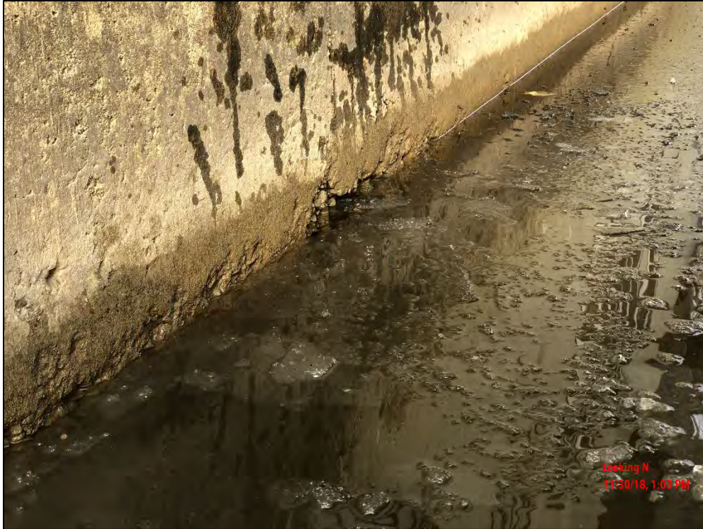
Photo 23: Previously visible, now fully submerged, spalled area approximately 10'-0" north of the south end of the West pier's east face.
