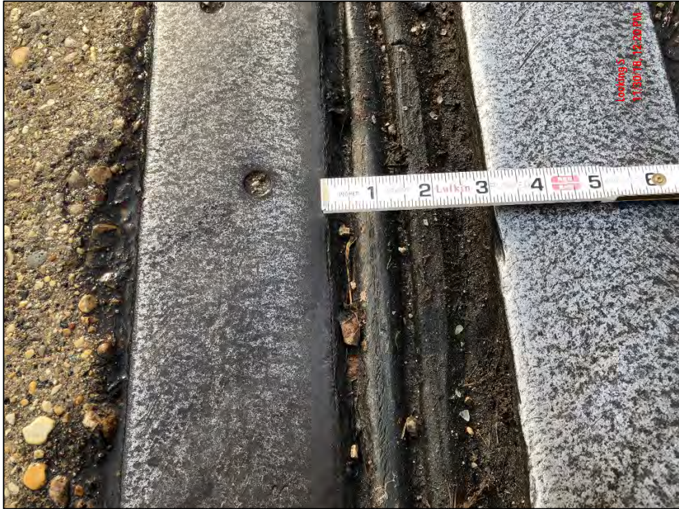
Photo 5: East abutment expansion joint measuring 3" opening with a 1" settlement. Joint glands have failed causing leakage to the abutment at areas without any debris.
