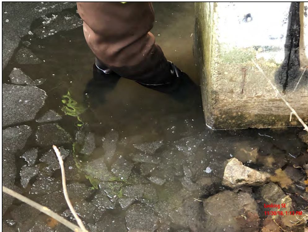
Photo 22: Undermining noted at the north end of the West pier.
