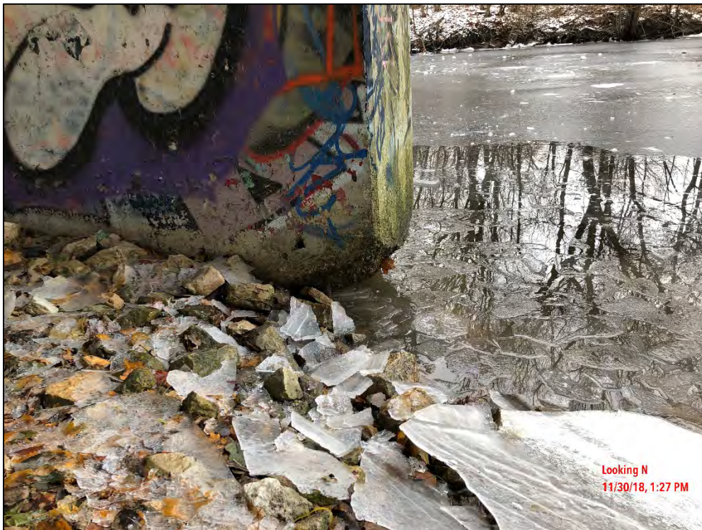
Photo 26: Deep spall at the north end of the East pier measuring 3' depth x full width x 2'.
