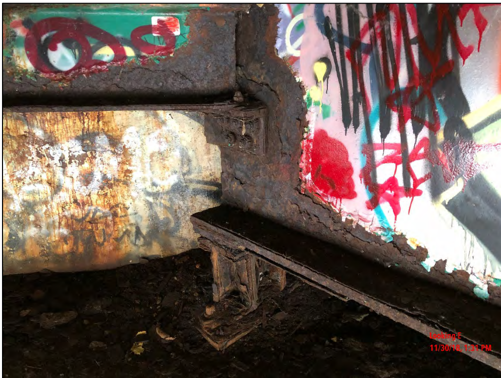
Photo 18: Typical beam and bearing corrosion at East abutment.
