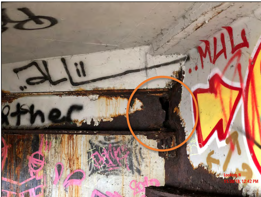
Photo 12: Complete section loss at beam 3 and diaphragm, at the north end at the west abutment.
