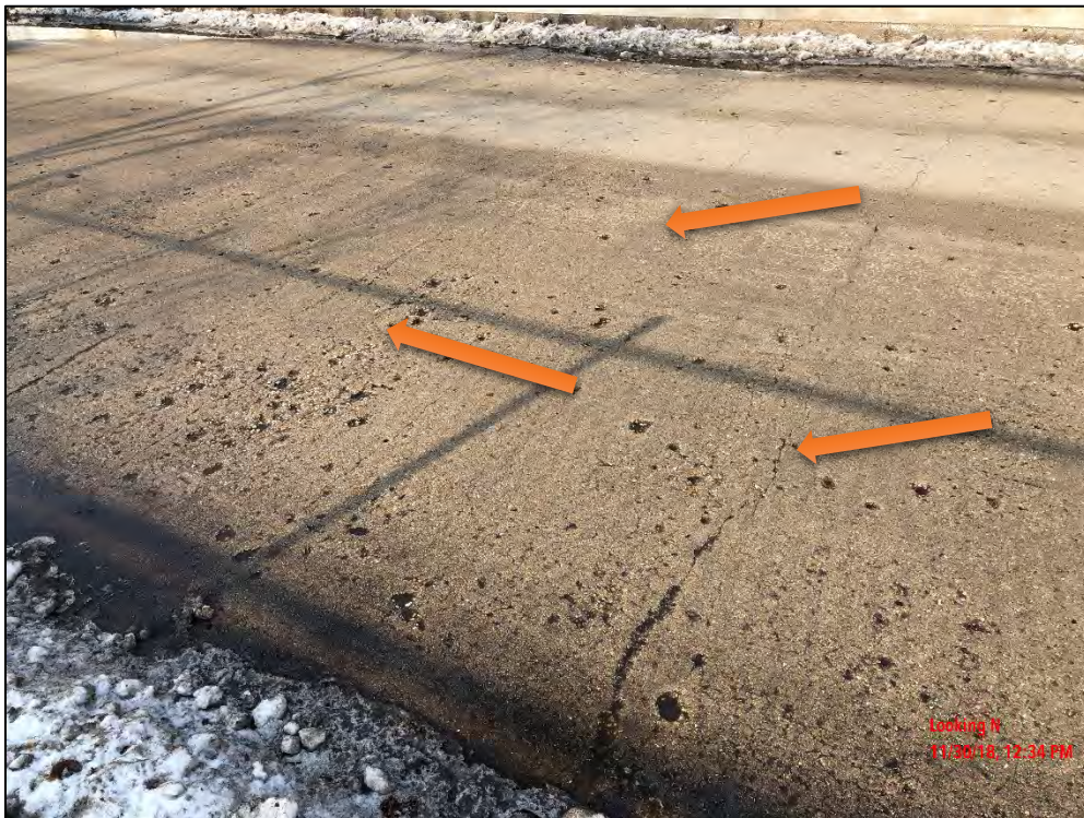
Photo 4: Full width transverse cracks noted at 30 inches centers.
