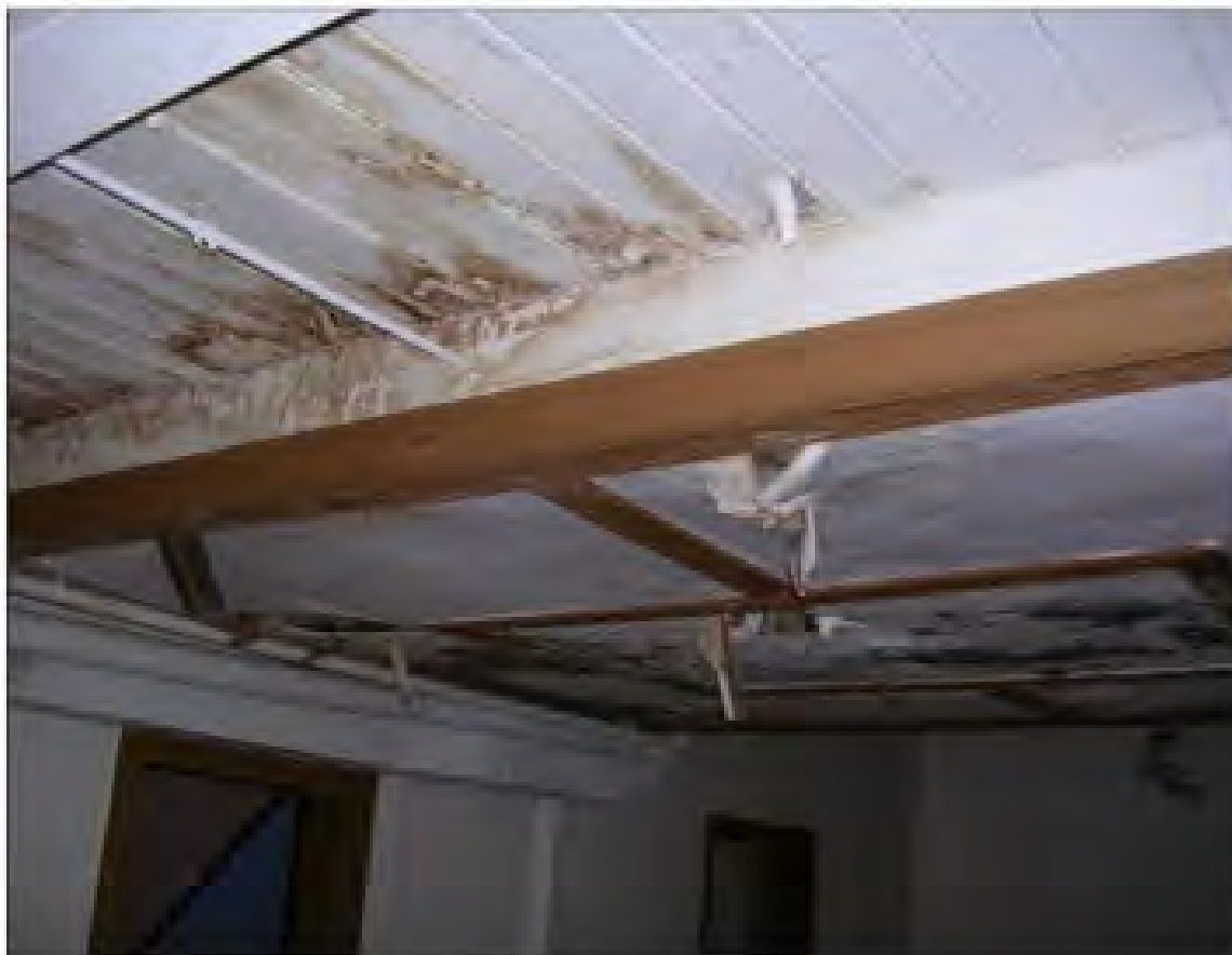
Photograph 8 – Another view of suspect mold located on the first floor of the building.
