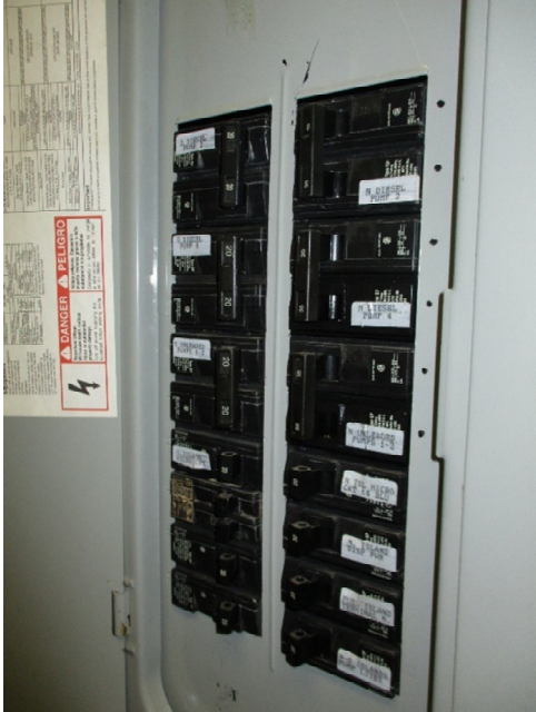
Figure 4: EM panel located in utility closet
