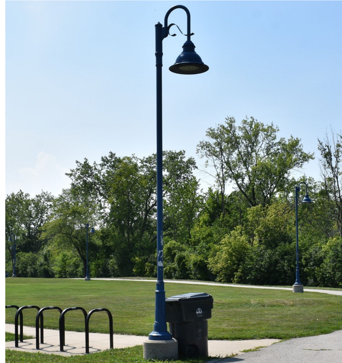
Security lighting - Twiggs Park
