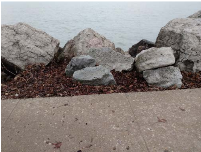
Image 3: Section loss in crest protection
