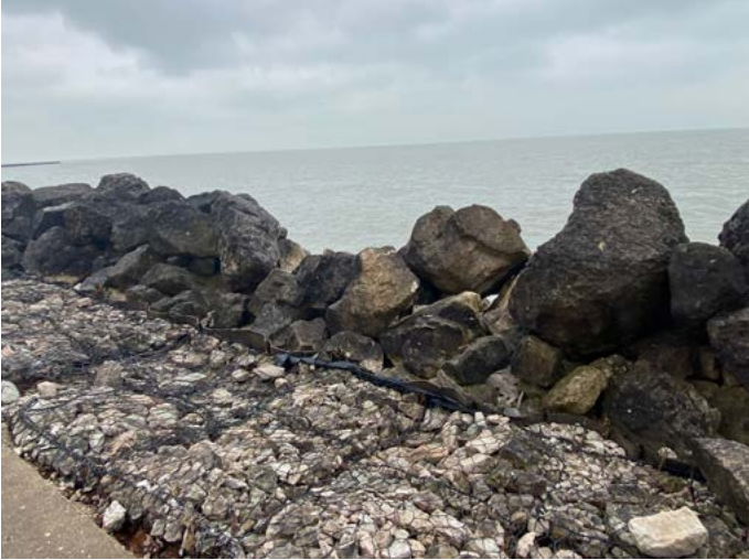
Image 2: Section loss in revetment crest
