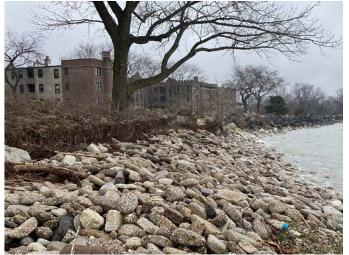
Image 2: Significant erosion at embankment
