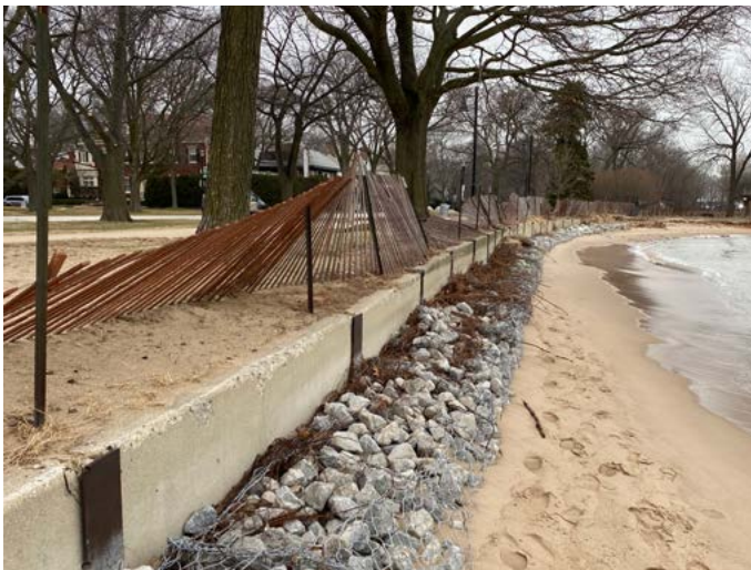
Image 3: Damaged gabions along wall
