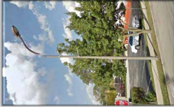
COBRA HEAD INDUCTION (ROADWAY)
