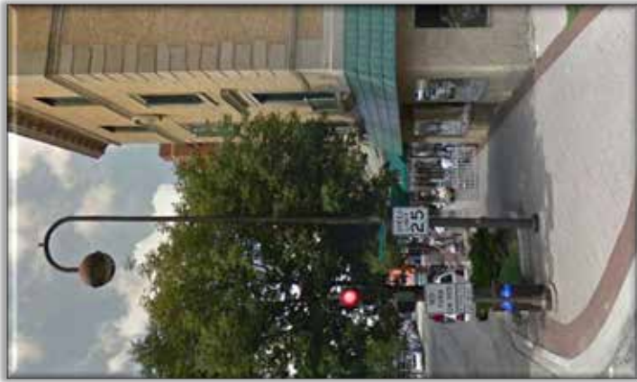
GLOBE TYPE METAL HALIDE (ROADWAY)
