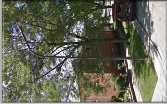
COBRA HEAD METAL HALIDE (ROADWAY)
