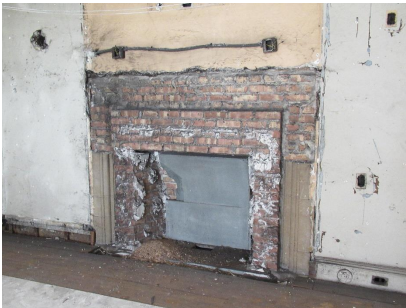
Figure 42. Fireplace with trim and tile missing
