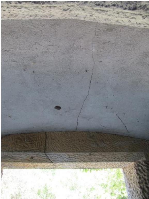
Figure 32. Cracked ceiling at entrance porch
