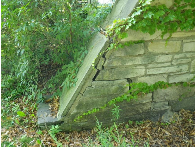
Figure 21. Wing wall at northwest corner of mansion (2016)
