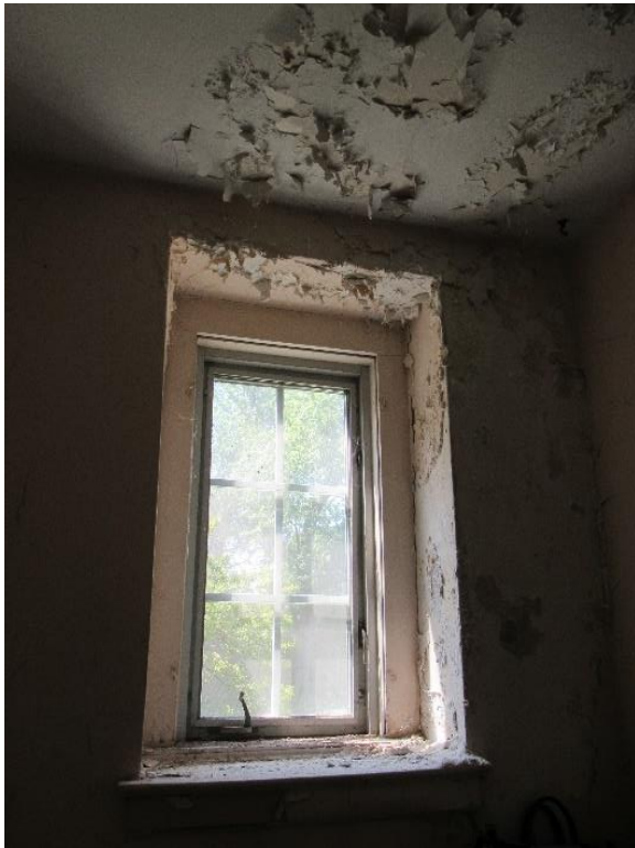
Figure 58. Water damage plaster adjacent to windows
