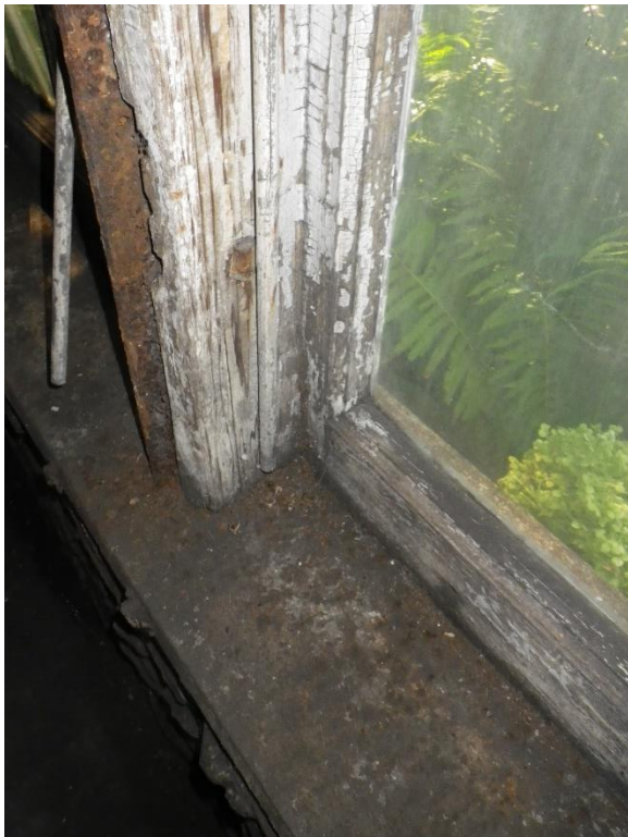
Figure 50. Deteriorated window sill and jamb in conservatory (2016)
