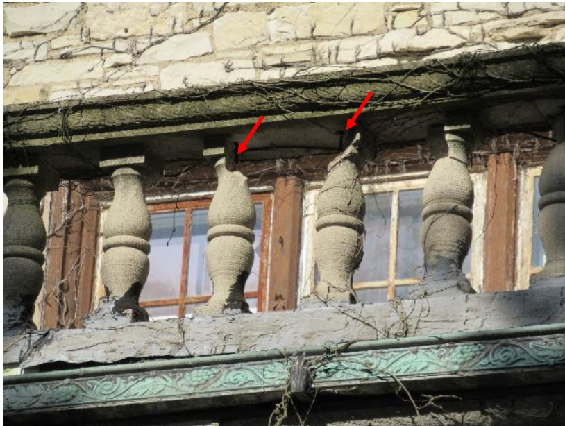
Figure 24. Spalled balusters above sun room
