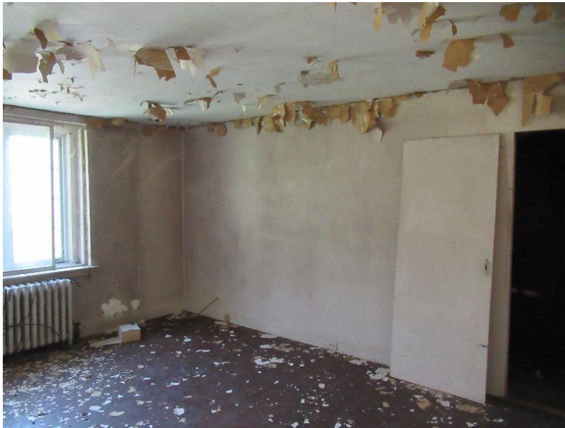
Figure 56. Peeling paint throughout interior of coach house
