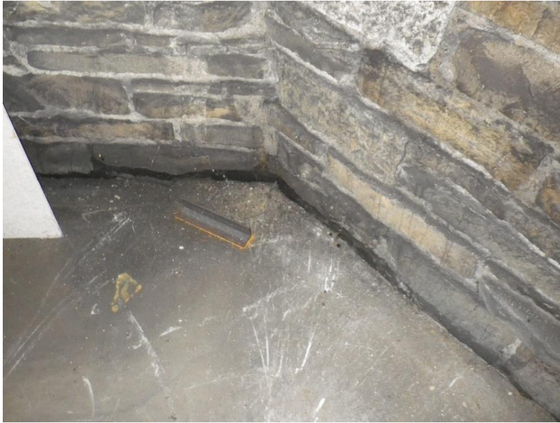
Figure 51. Deterioration of stone on interior of conservatory (2016)
