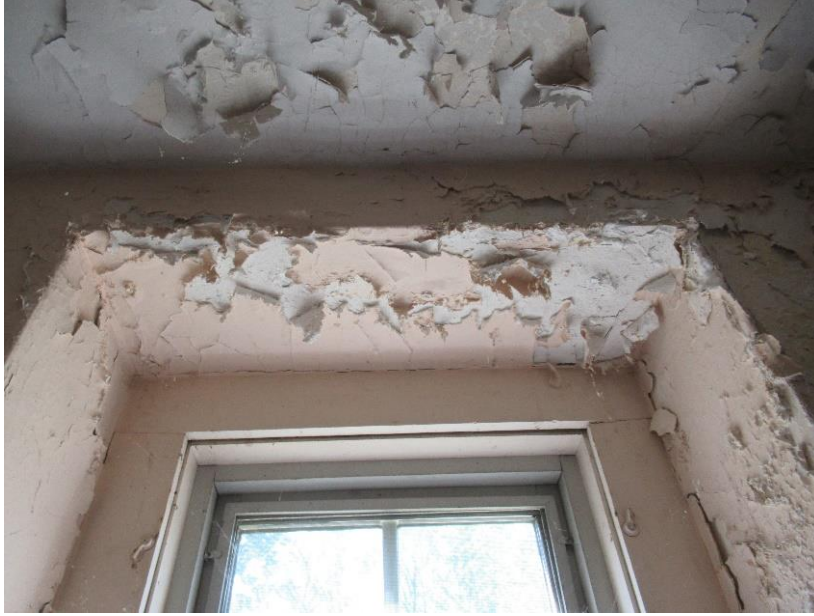
Figure 59. Water damage plaster adjacent to windows
