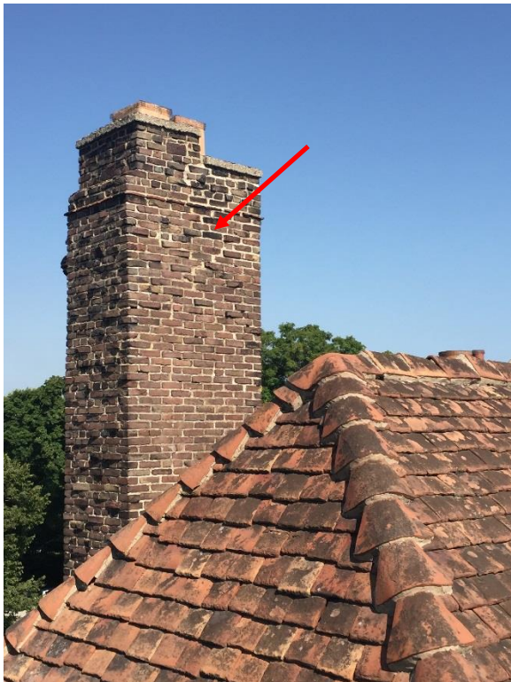
Figure 28. Isolated cracking in chimney (2016)
