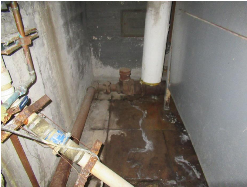
Figure 46. Basement mechanical room with standing water
