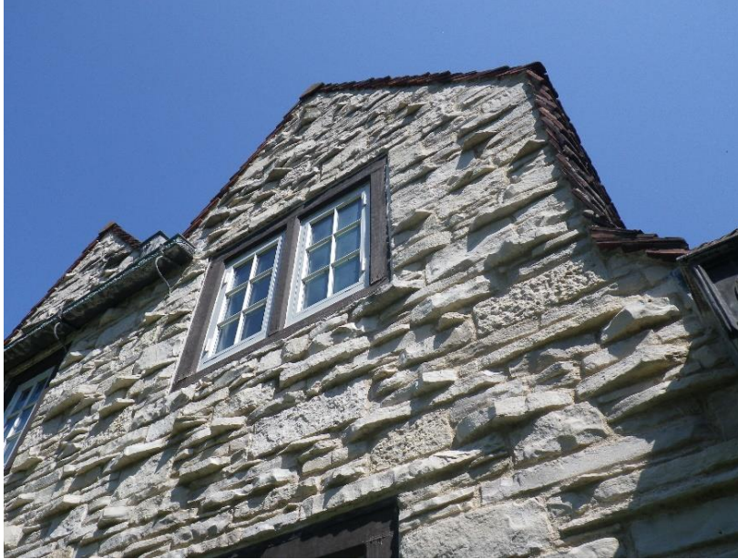
Figure 55. Second floor window on south facade of coach house. Windows appear to be replacement aluminum or aluminum clad casement units set in the original wood window surround (2016)
