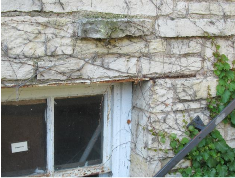
Figure 33. Surface corrosion of window lintel
