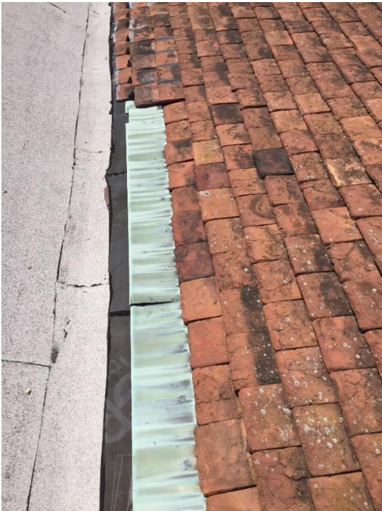
Figure 36. An area of missing roof tiles (2016)
