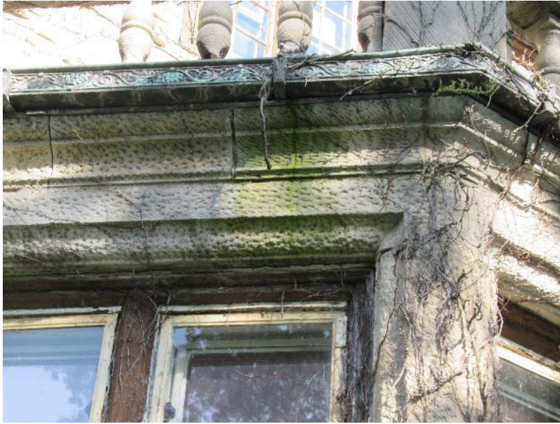
Figure 23. Cracking of limestone cladding at sun room and algae staining
