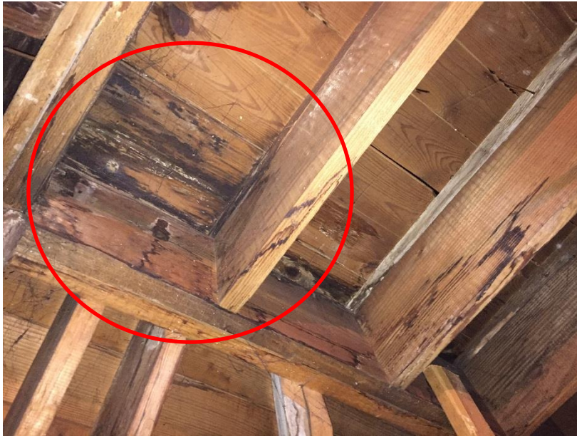
Figure 47. Water staining on wood framing members (2016)
