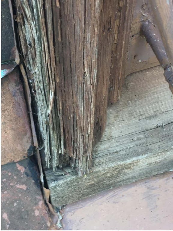
Figure 39. Checks at wood door trim at fire escape (2016)
