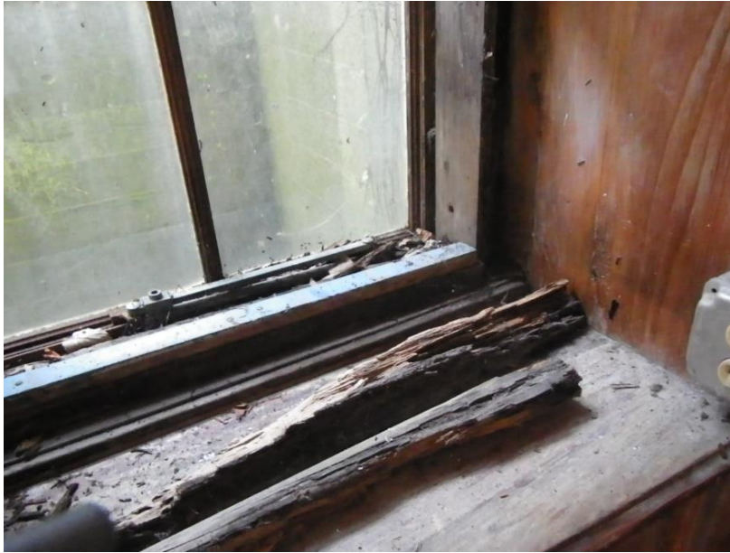
Figure 31. Deterioration wood sill in basement (2016)
