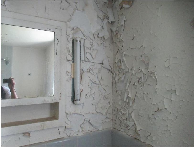
Figure 57. Peeling paint throughout interior of coach house
