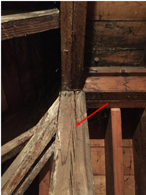
Figure 48. Checks in wood framing members (2016)
