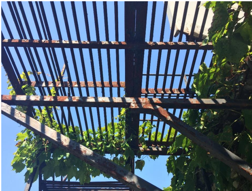
Figure 38. Surface corrosion and peeling paint and areas at the fire escape (2016)
