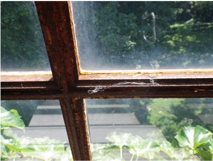
Figure 30. Surface corrosion on steel window mullions (2016)
