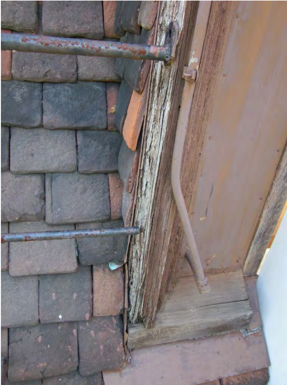
Photo 6 – Deteriorated wood trim at south fire escape exit doors.
