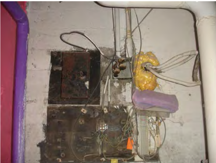
Old electrical open boxes
