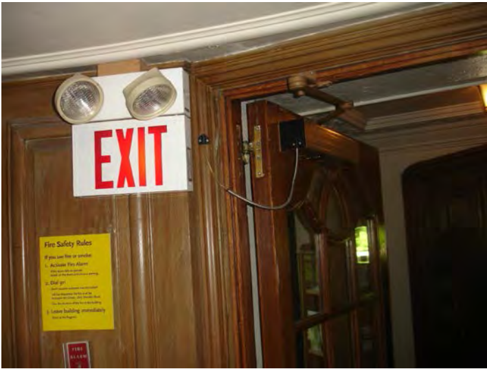
Accessible entrance not working
