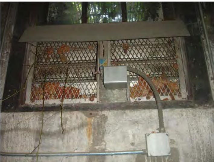
Combustion air intake for boiler room
