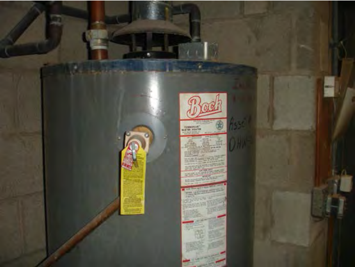
Domestic hot water heater
