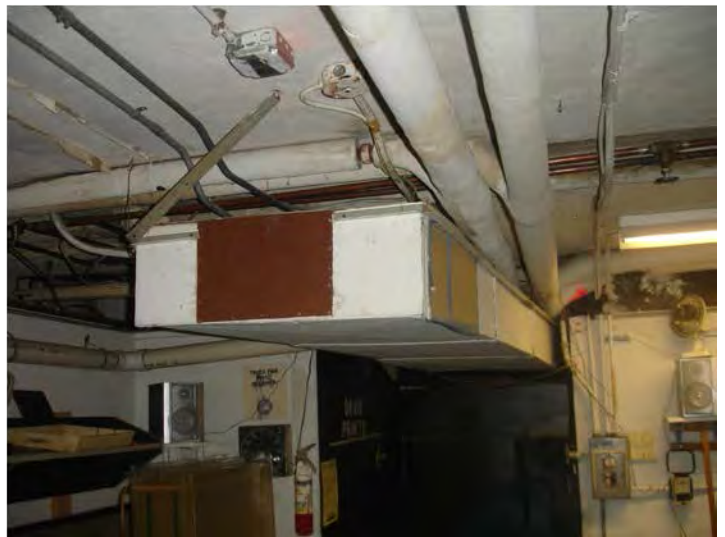
Photo lab blanked off grilles
