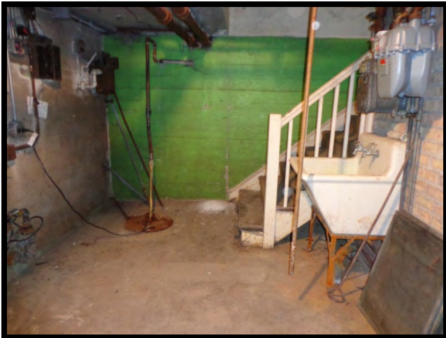
SUMP AND FUEL OIL UST GAUGE IN THE BASEMENT OF THE COACH HOUSE
