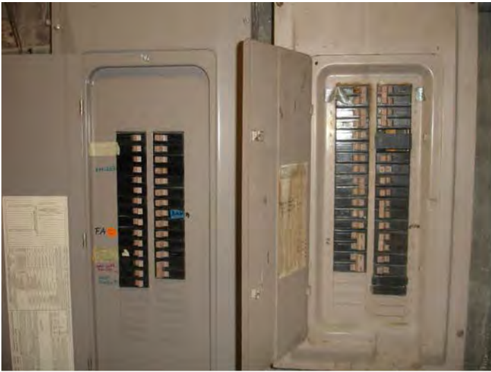
Older electric panels
