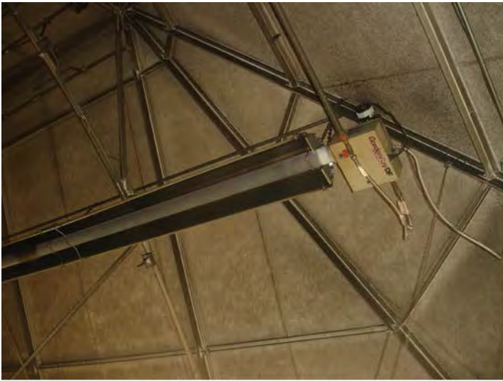
Metal shop heating unit
