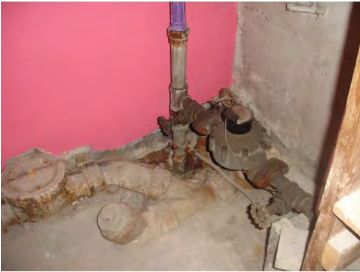
Incoming water service
