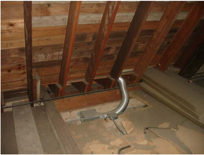
3rd floor toilet exhaust ducted through attic
