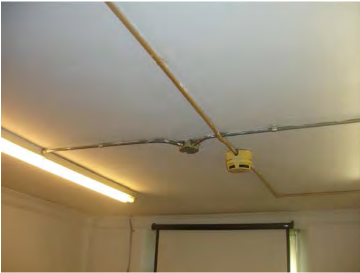
Ceiling of 3rd floor office
