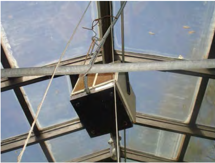
Green house heating unit
