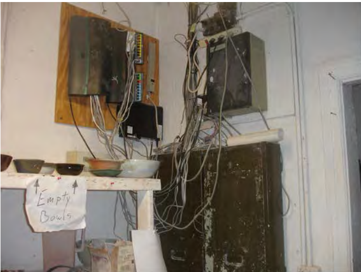
Old telephone and open electrical boxes
