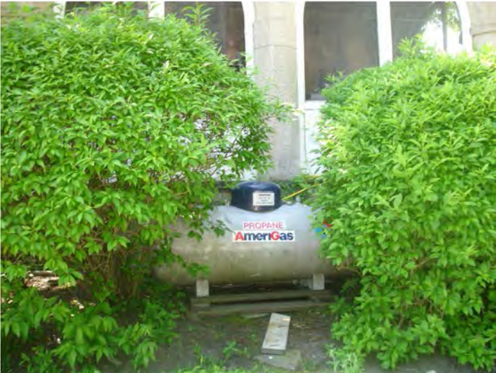
Propane tank on grade
