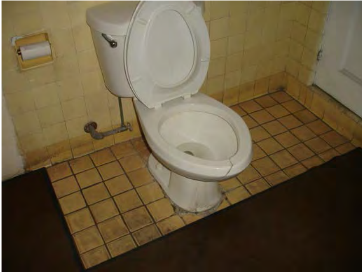
3rd floor toilet room (fixture cracked)
