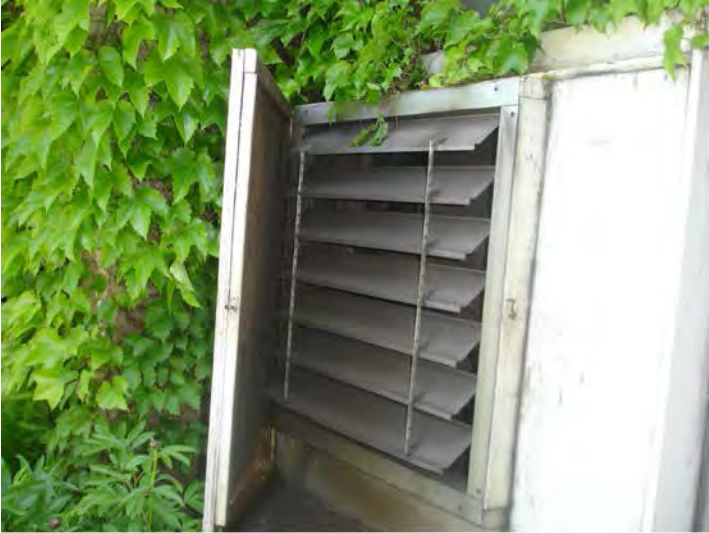
Spray booth exhaust
