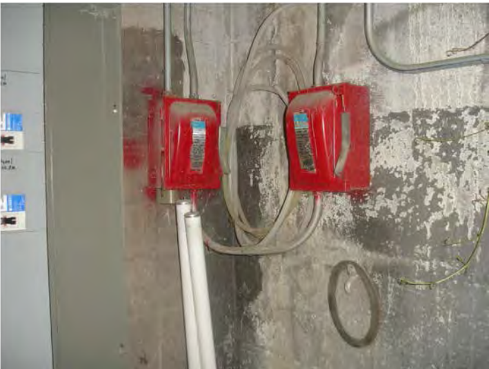
Emergency power switches
