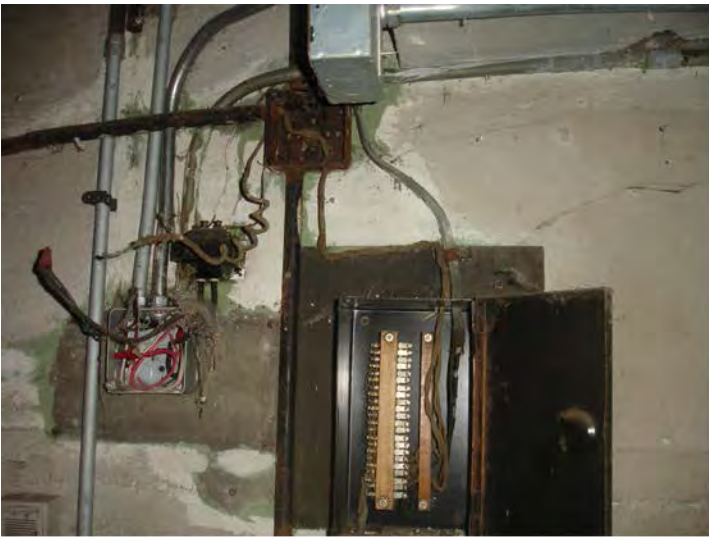
Old electrical panel
