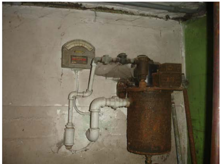
UG tank level equipment (abandoned)
