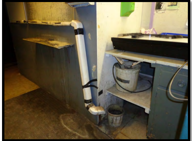
PHOTO VIEWING AREA WITH STAINING ON THE FLOOR
