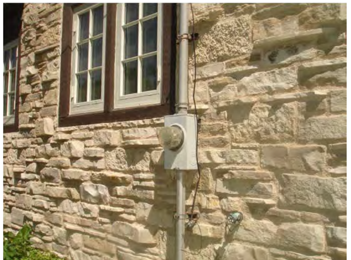
Coach house electric meter
