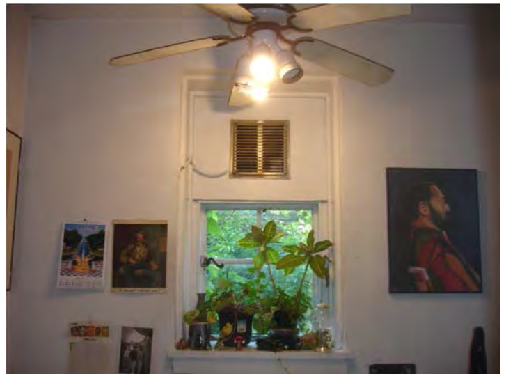
Office with exhaust
