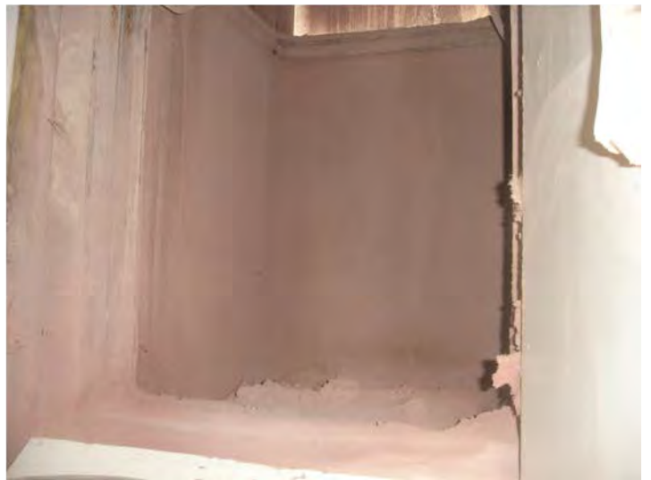
Spray booth exhaust
