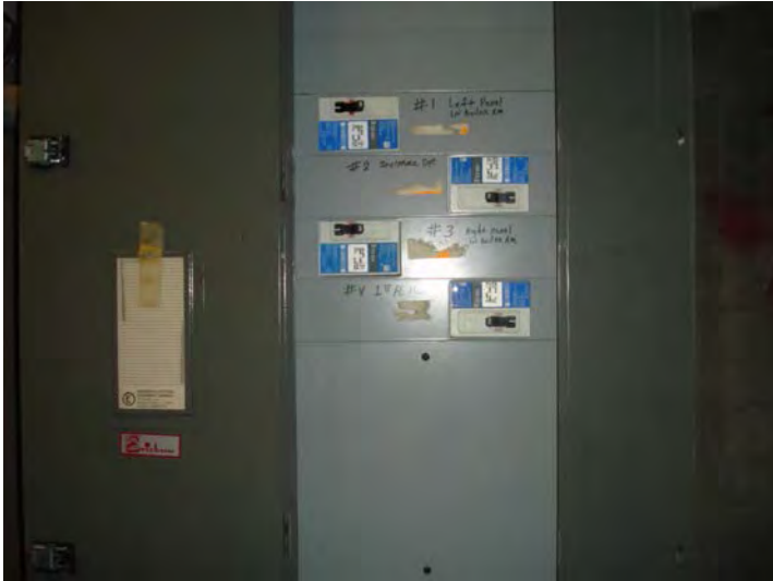
Main electrical panel
