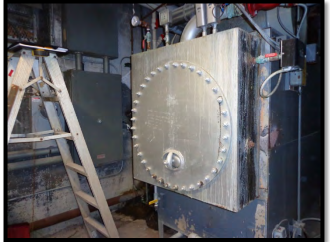
BOILER ROOM IN THE BASEMENT OF THE MAIN BUILDING
