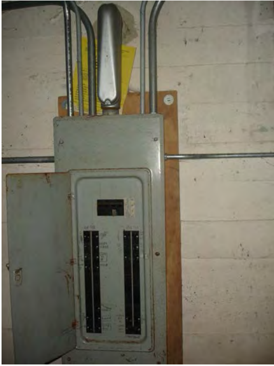
New coach house electrical panel
