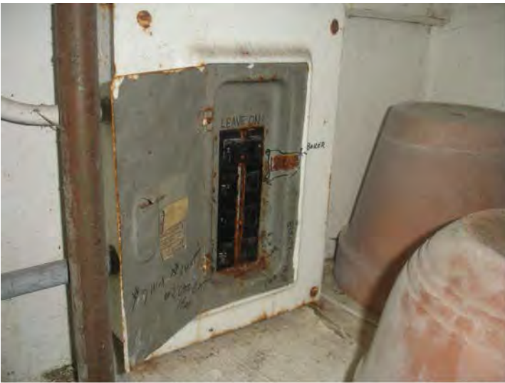
Green house electrical panel
