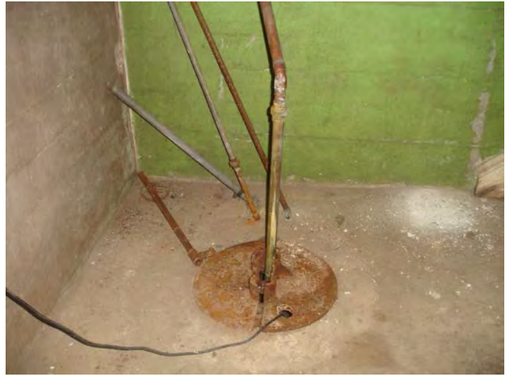
Sump pump in basement of coach house
