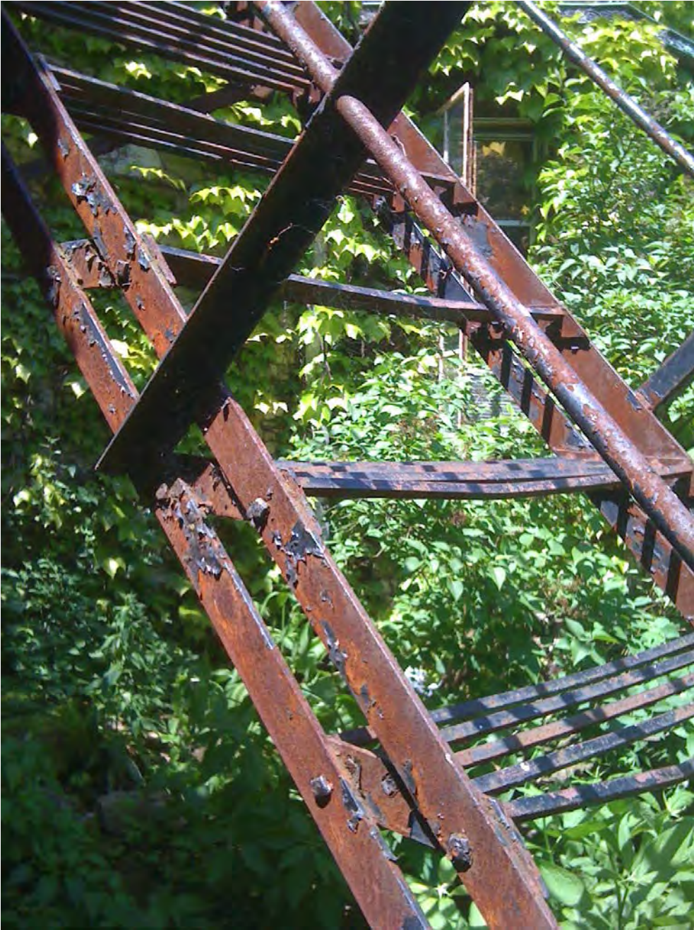
Photo 8 – Surface corrosion and tread deterioration on fire escape.
