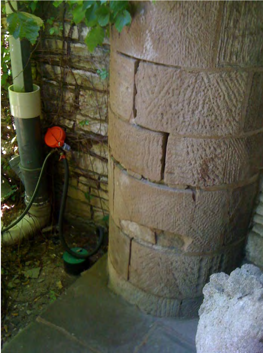
Photo 3 – Mortar deterioration at west porch
