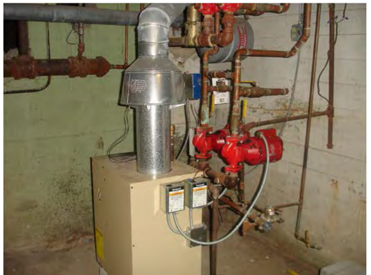
Boiler in coach house basement
