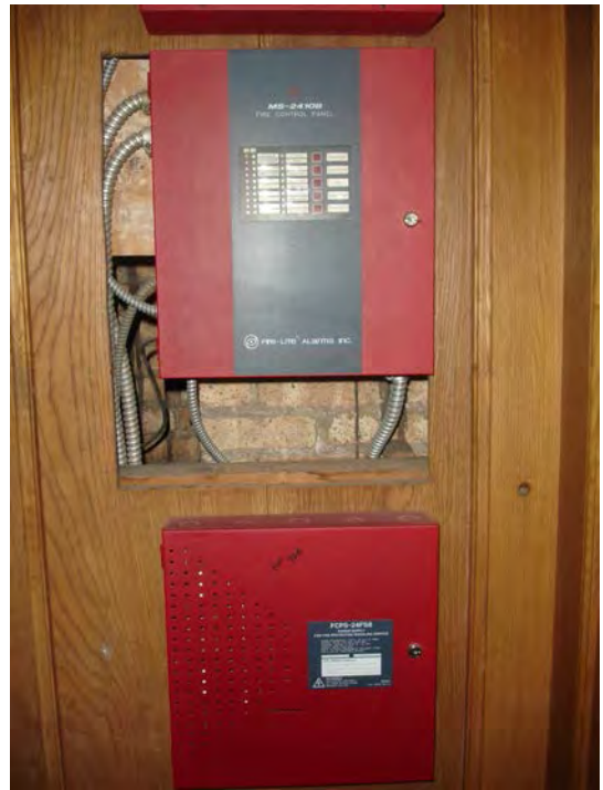
Fire alarm panel
