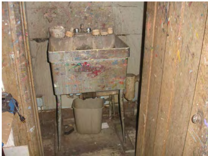
Slop sink in 3rd floor art studio
