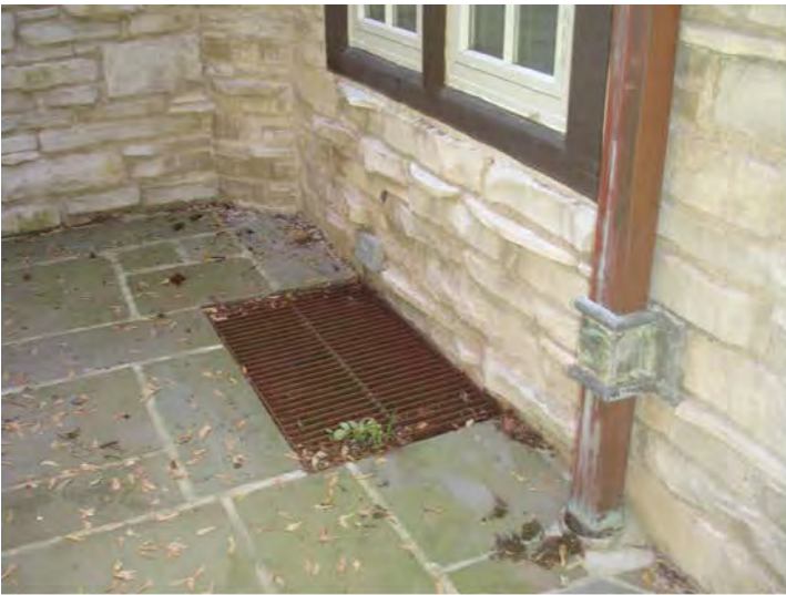
Combustion air to basement
