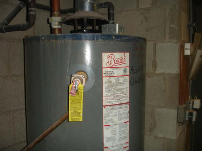
Domestic hot water heater
