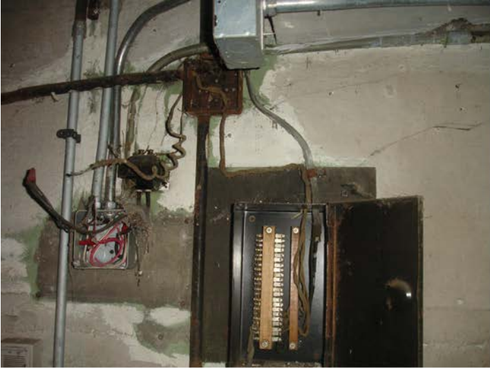
Old electrical panel
