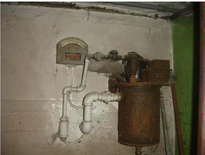
UG tank level equipment (abandoned)
