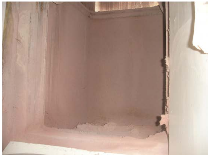
Spray booth exhaust
