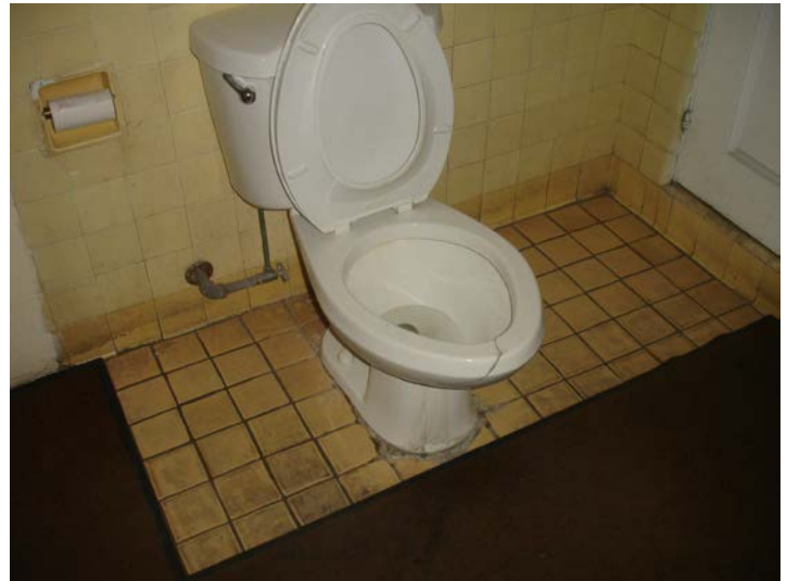
3rd floor toilet room (fixture cracked)
