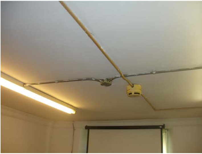
Ceiling of 3rd floor office
