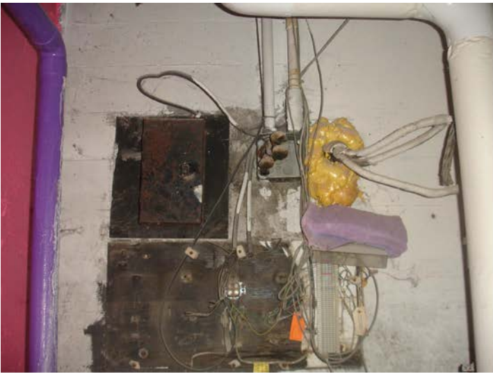
Old electrical open boxes
