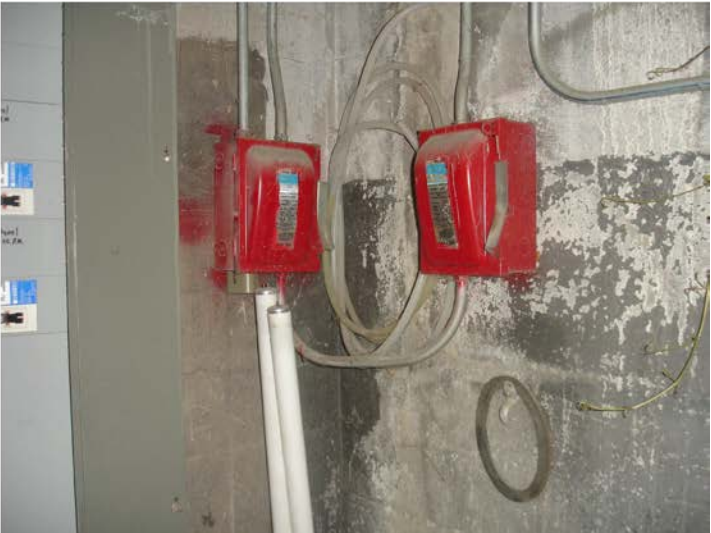
Emergency power switches
