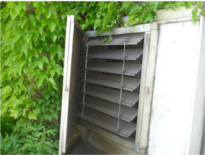
Spray booth exhaust
