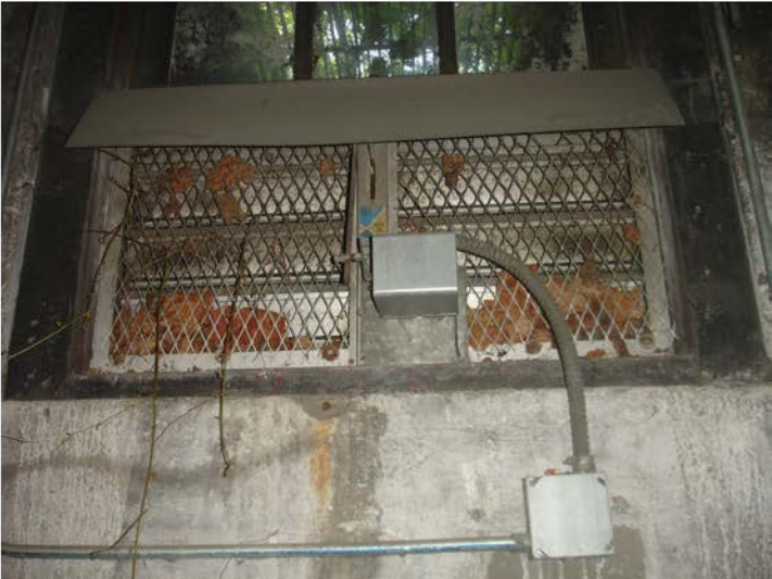
Combustion air intake for boiler room
