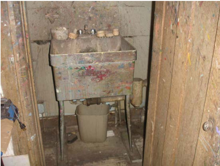
Slop sink in 3rd floor art studio
