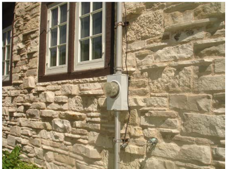
Coach house electric meter
