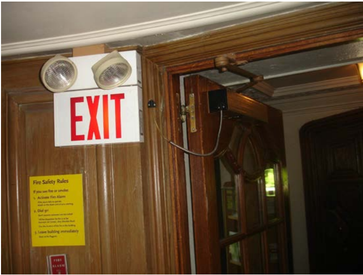
Accessible entrance not working
