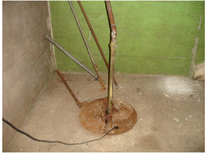
Sump pump in basement of coach house
