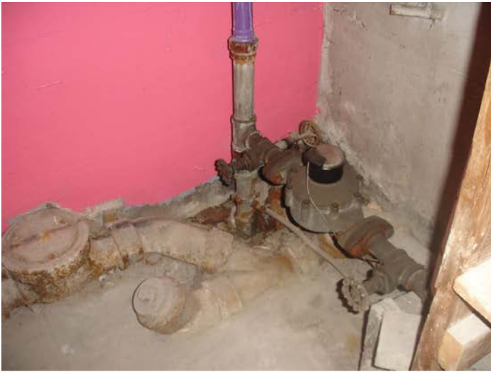
Incoming water service
