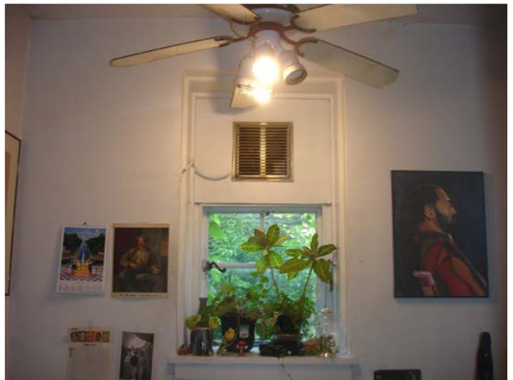
Office with exhaust
