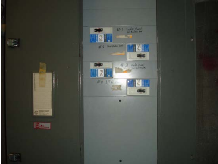
Main electrical panel
