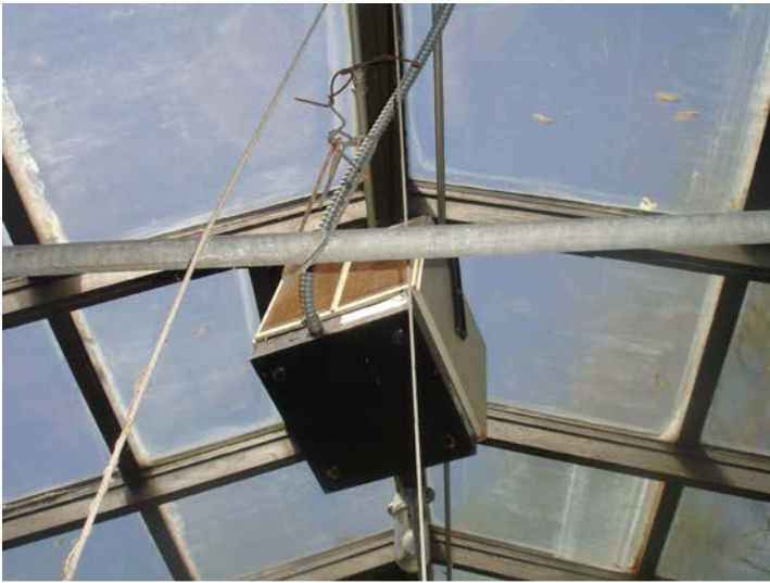
Green house heating unit
