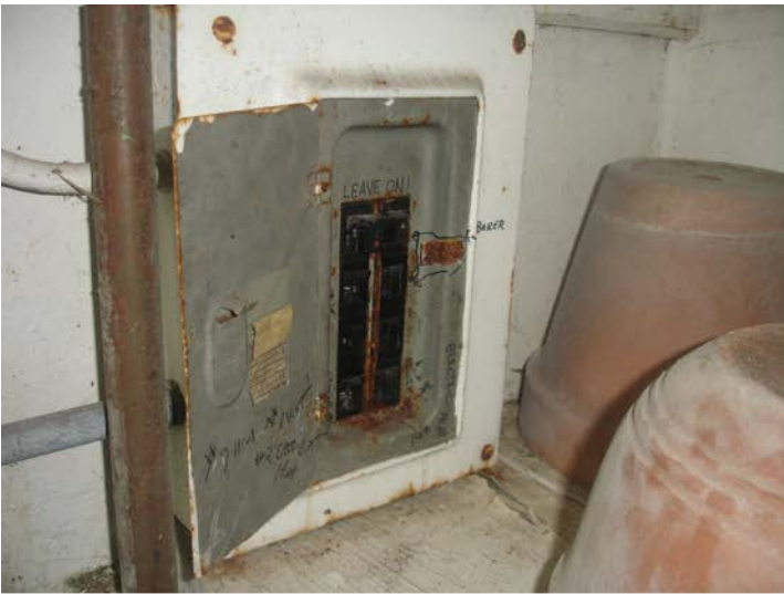
Green house electrical panel
