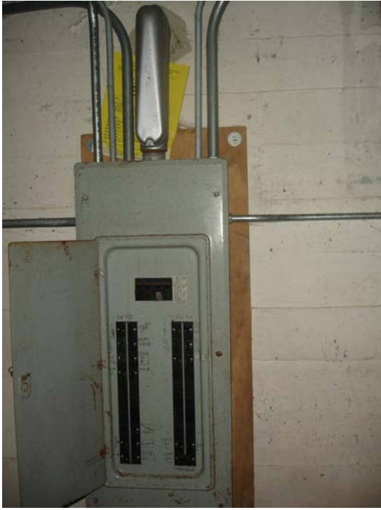
New coach house electrical panel
