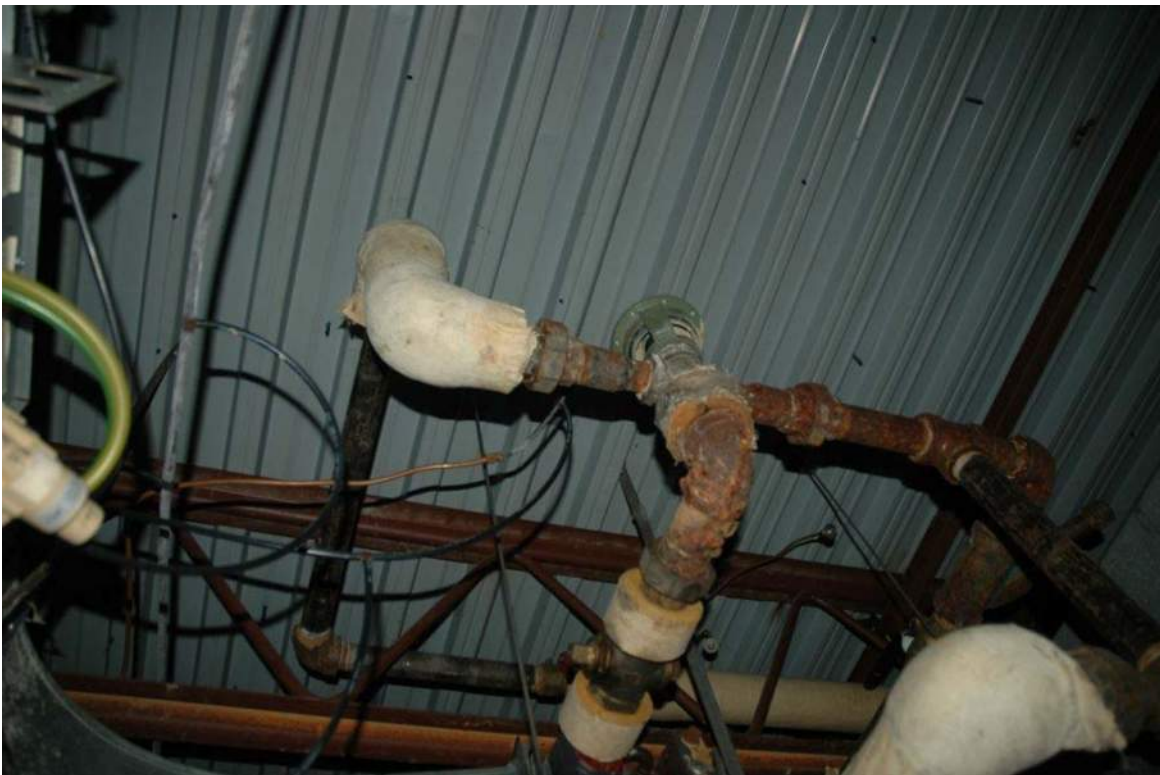
Mudded Elbow Insulation within Mechanical Areas
