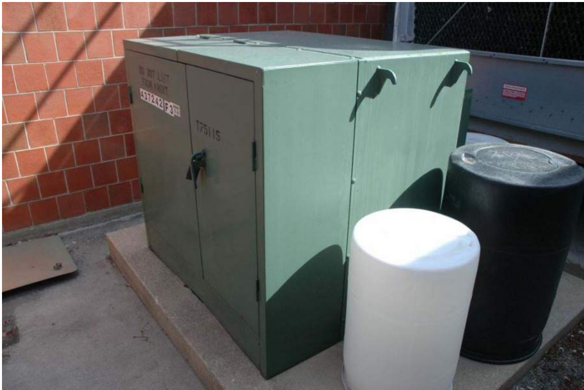
ComEd Electrical Transformer
