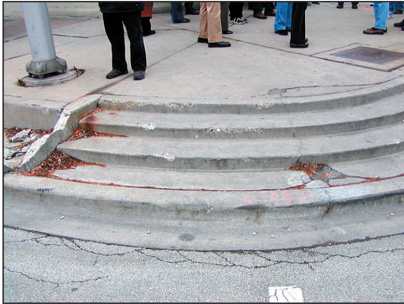
Steps and deteriorated sidewalk conditions at Green Bay Road.
