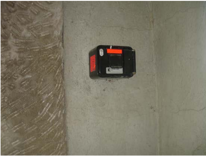
Knox box at entrance
