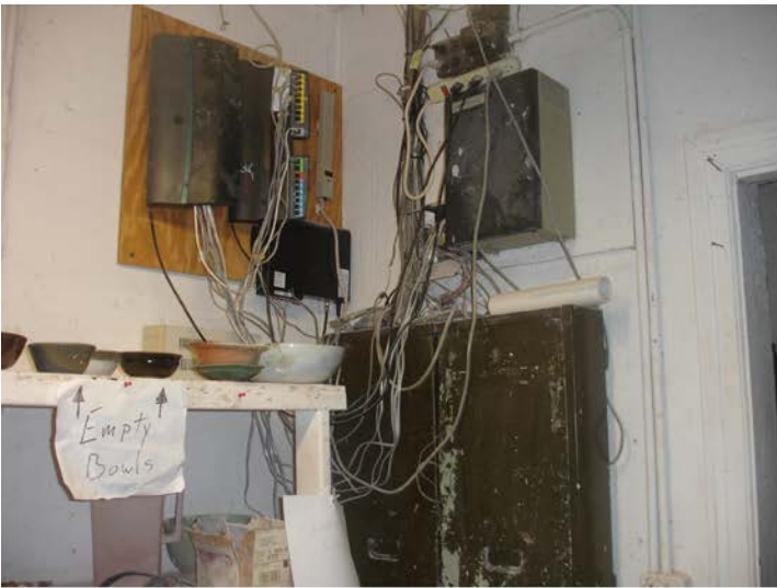
Old telephone and open electrical boxes
