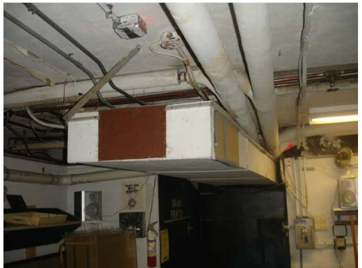
Photo lab blanked off grilles
