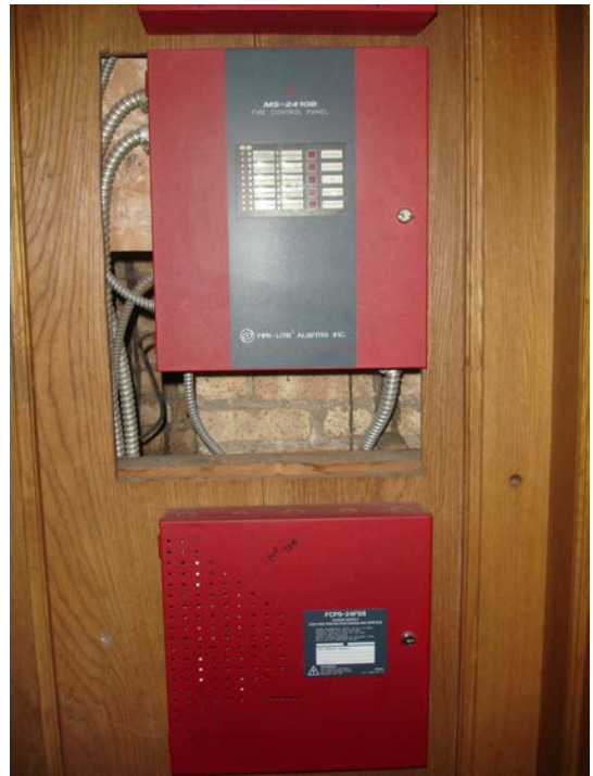
Fire alarm panel
