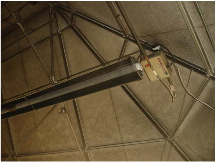
Metal shop heating unit
