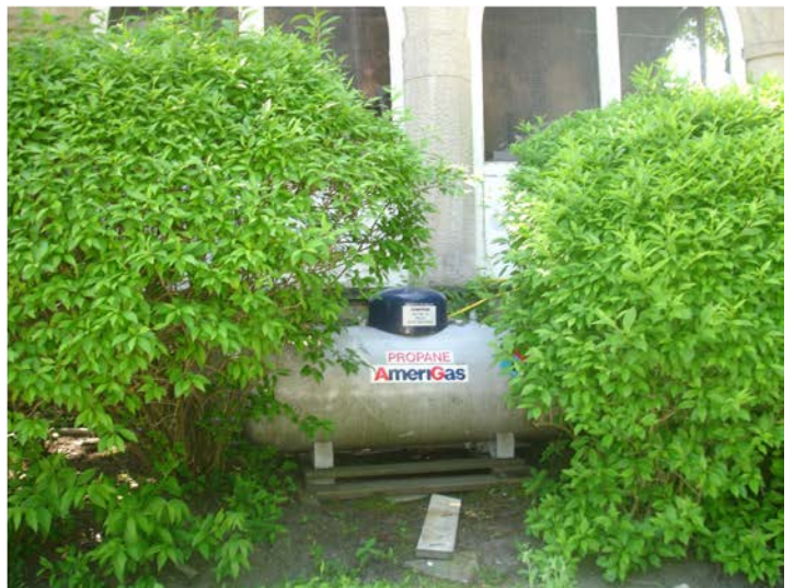
Propane tank on grade
