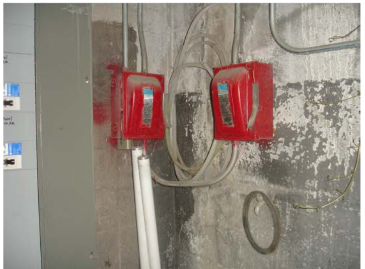
Emergency power switches
