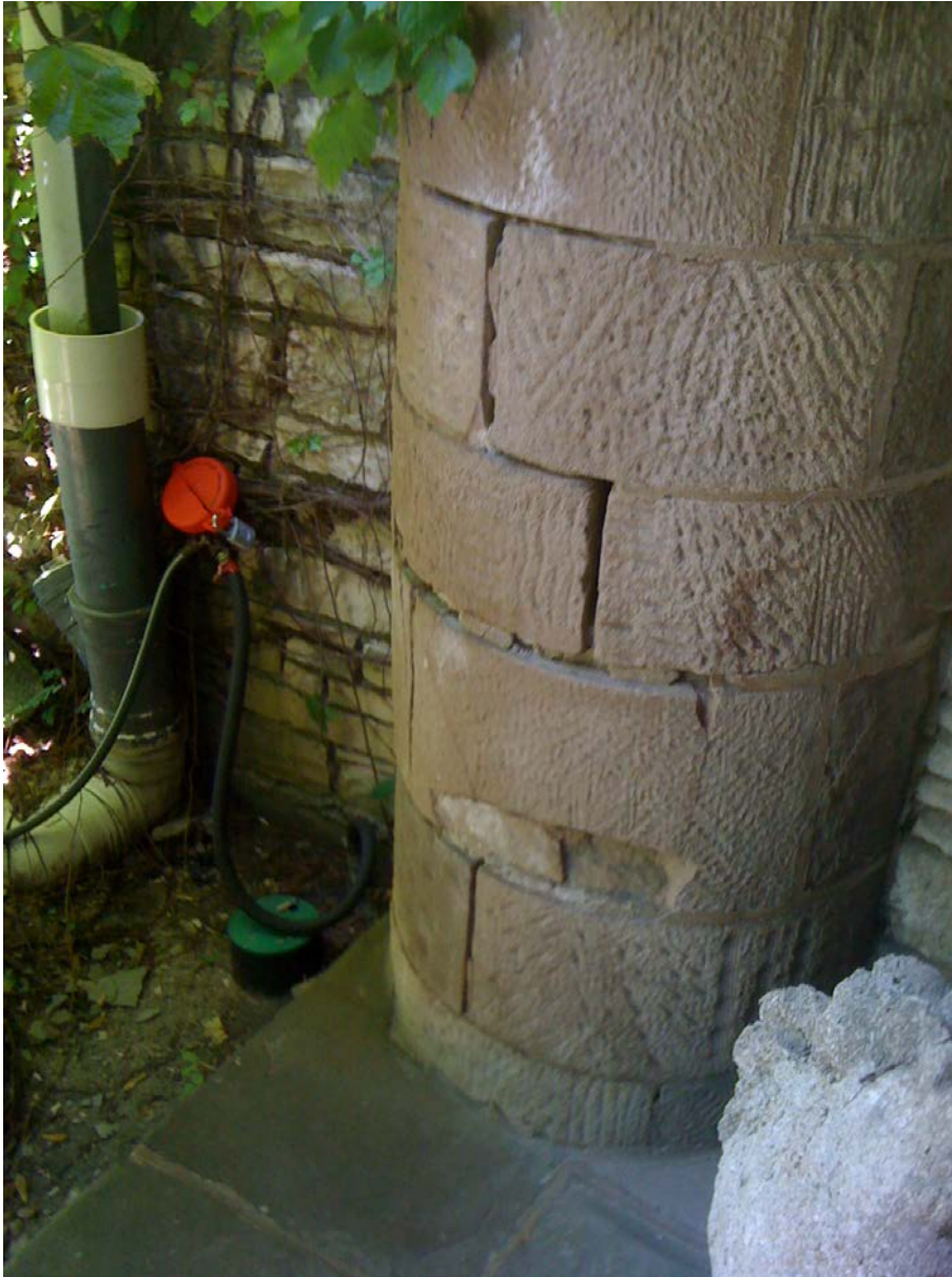
Photo 3 – Mortar deterioration at west porch
