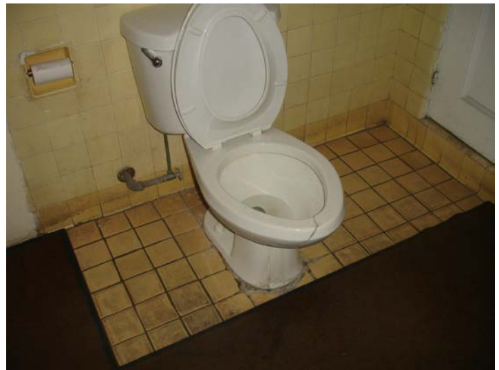
3rd floor toilet room (fixture cracked)
