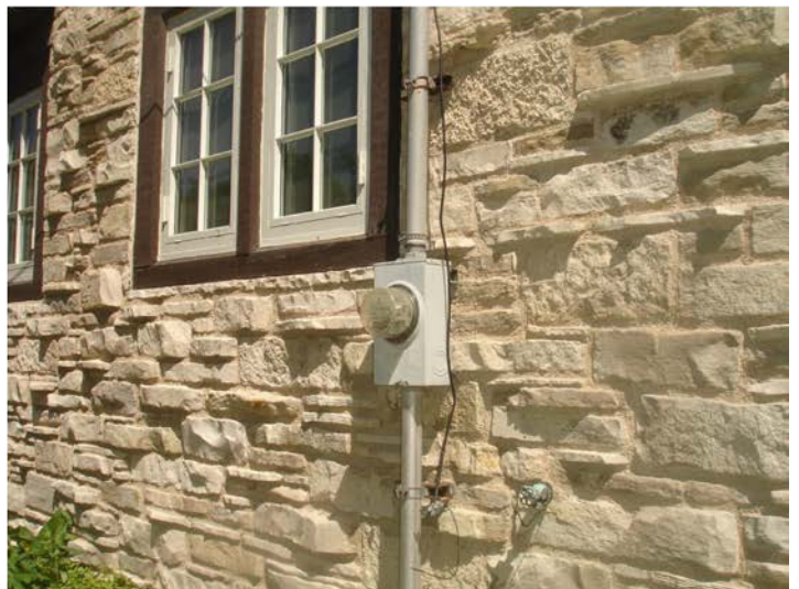
Coach house electric meter
