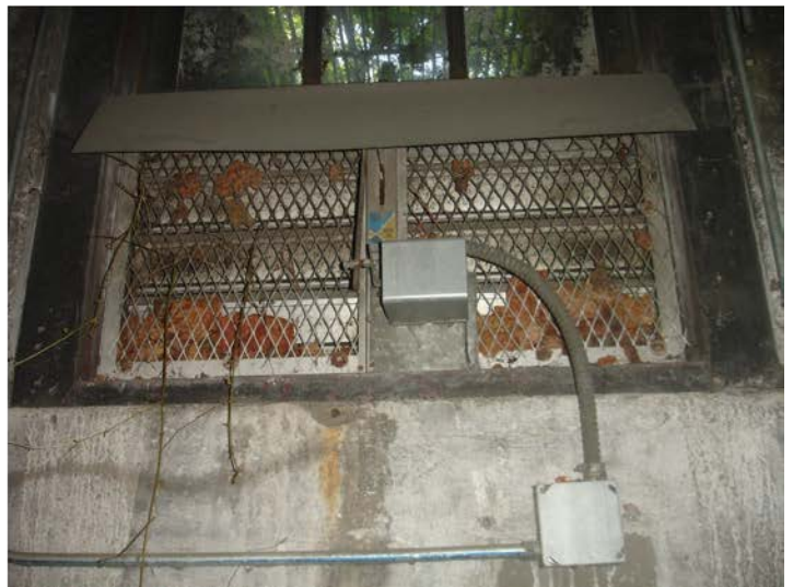
Combustion air intake for boiler room
