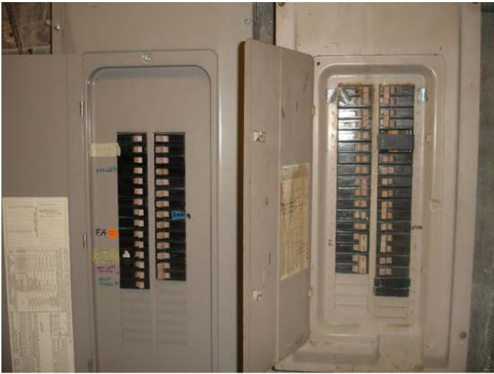
Older electric panels
