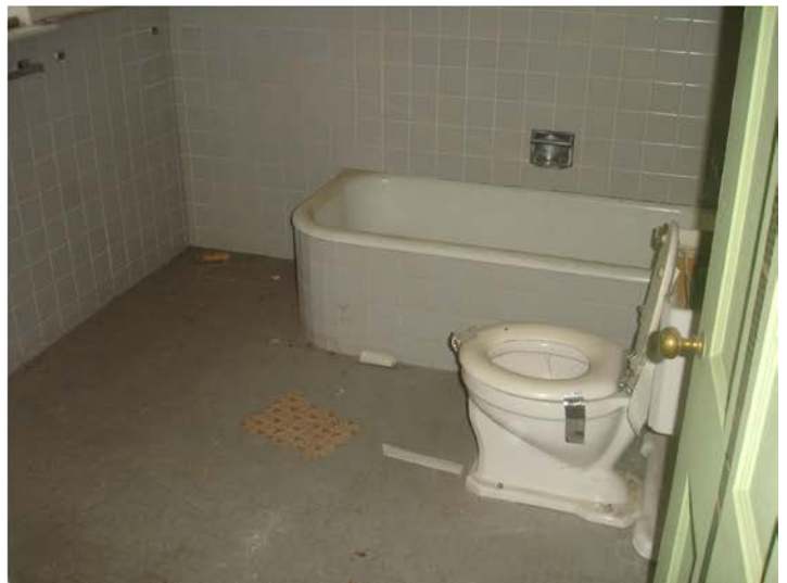
Coach hose apt. toilet room
