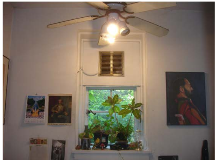
Office with exhaust
