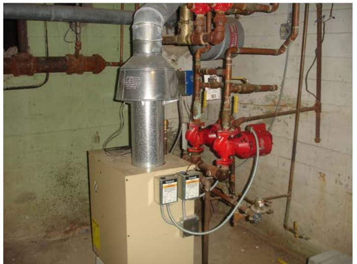
Boiler in coach house basement
