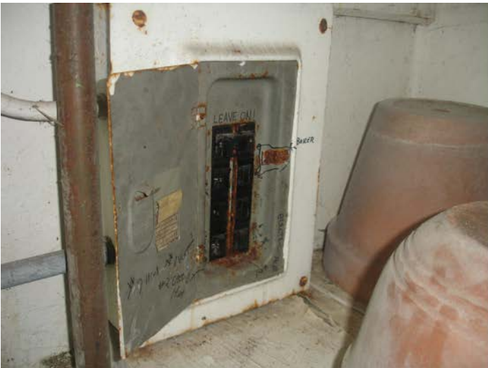
Green house electrical panel
