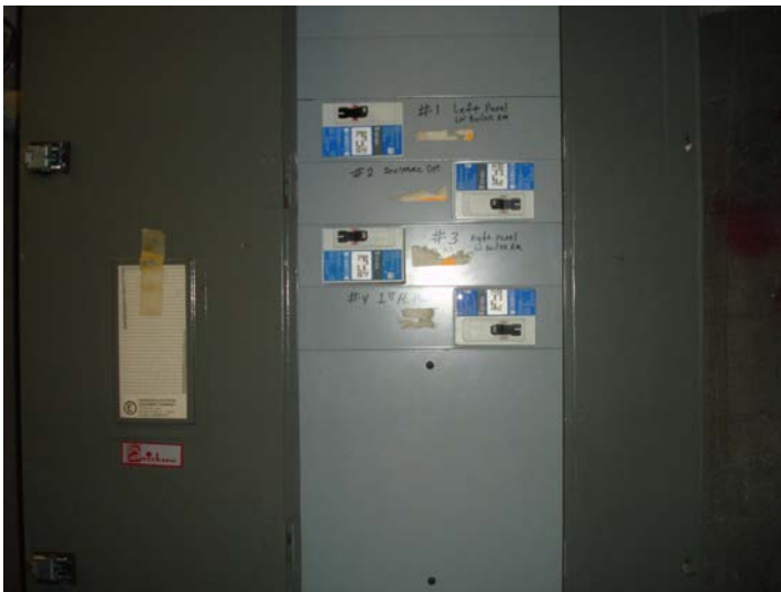
Main electrical panel
