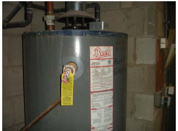
Domestic hot water heater
