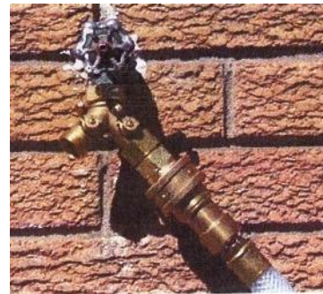
Y connector at outside hose spigot with temporary supply connected at right
