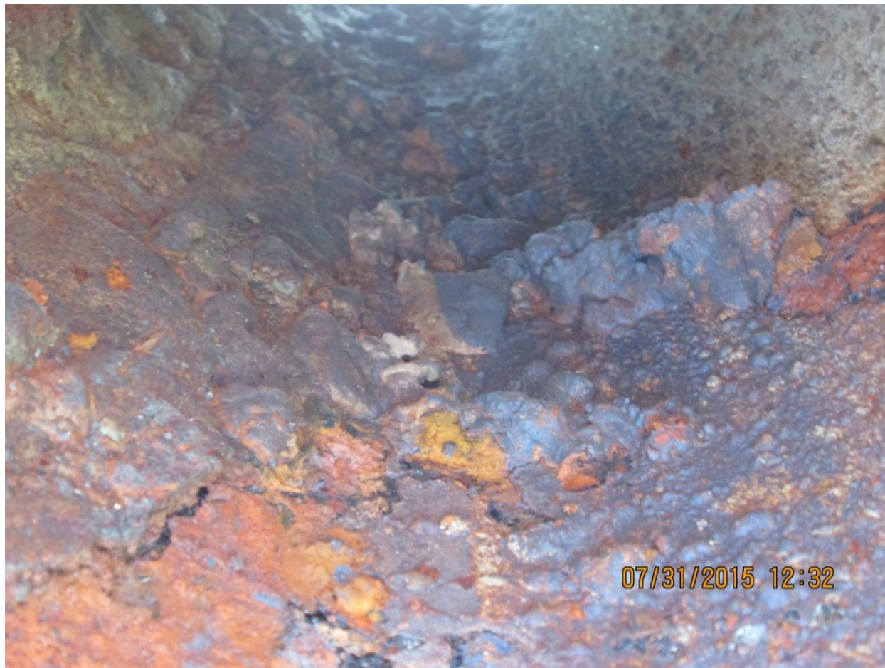
Figure 4 of the 2017 SCS PAR, Photograph 33, showing the friable Black Crust inside the Dodge Avenue Water Line
