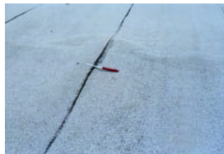
Photo R-10: View of a blister on Roof E.
