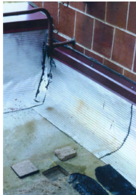
Photo R9: View of test cut #7 after removal of the membrane and perlite. Water may have migrated from the wall cracks (upper center).
