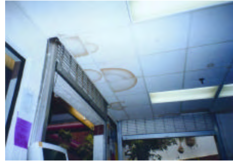
Photo R-3: View of stained ceiling boards in room A132.
