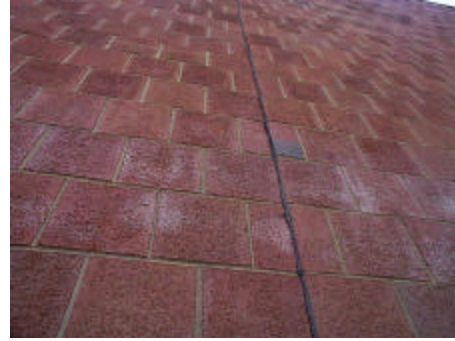
Photo S-4: Main Ice Rink – Eastern Wall – Bowed masonry wall.
