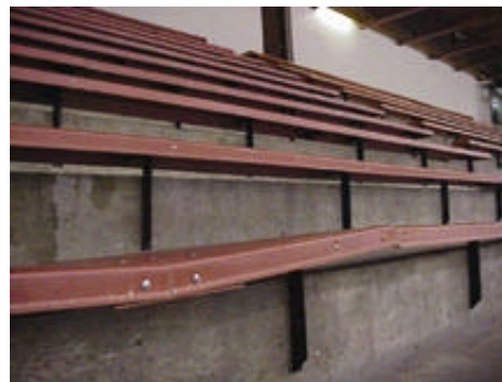
Photo A-10: Broken Bleacher Seats
