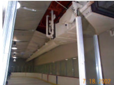
Photo M-1: Air handling unit in Skating Rink
