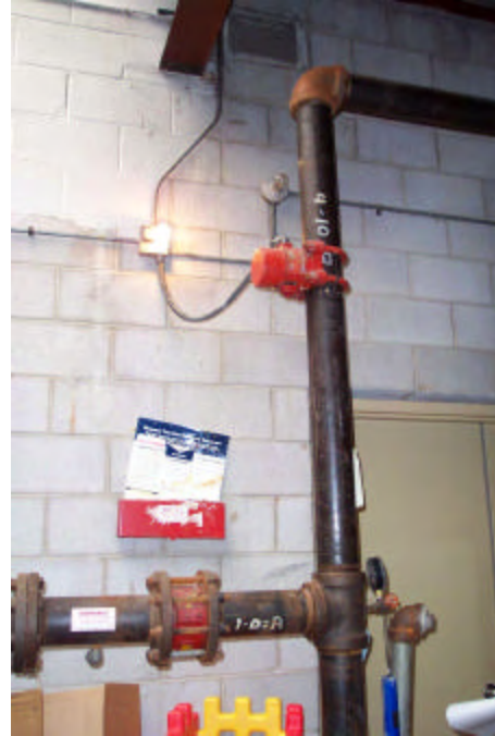
Photo FP-4: Waterflow switch on sprinkler riser.
