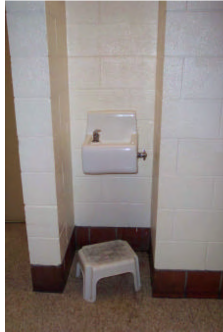
Photo P-4: Drinking fountain.
