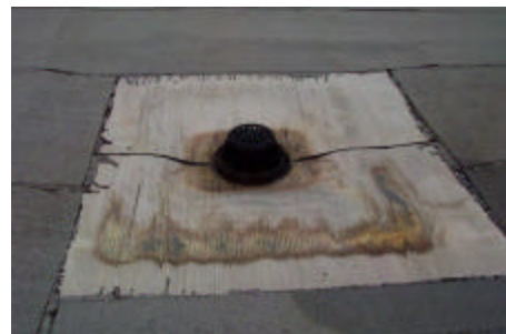
Photo P-6: Roof drain.
