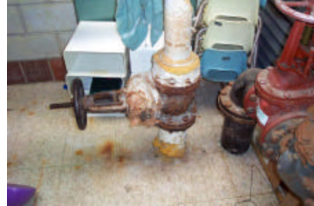
Photo P-1: Incoming water service.
