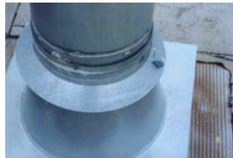
Photo R13: The storm collar was not sealed to the flue.
