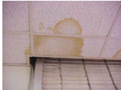
Photo A-13: Water Stained Ceiling Tiles at Office Area
