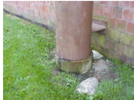
Photo A-3: North Side Drainage Condition
