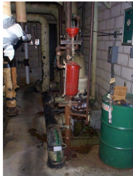
Photo RF-3: Circulating pumps.
