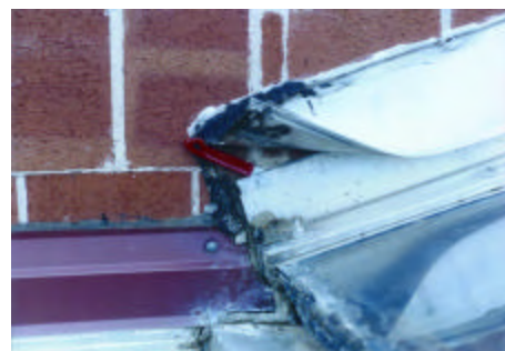
Photo R-16: View of the counterflashing at the main skylight. A putty knife is in the unsealed opening between the wall and the flashing leg.
