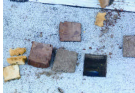
Photo R-4: Components left to right: Rigid fiberglass, phenolic, perlite, built-up membrane (above the perlite), sample opening, modified bitumen membrane.
