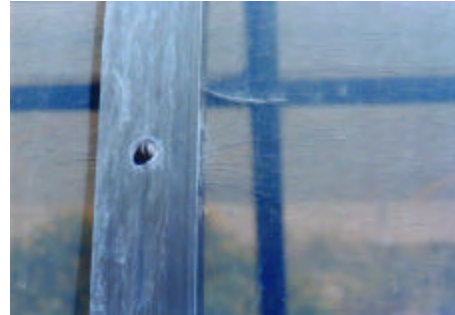
Photo R17: Close-up of crazed-crack glazing at the barrel vault skylight.
