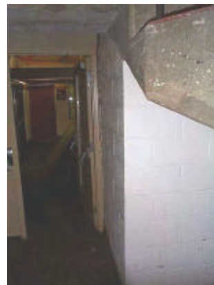
Photo S6: Main Ice Rink – Eastern End of Concrete Grandstand – Pinched doorframe.
