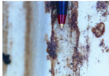
Photo R-7: Close up of test-cut #2, showing superficially corroded steel deck (the tip of the ink pen shows the scale of the photo).
