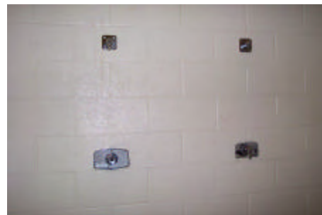
Photo P-5: Gang showers.
