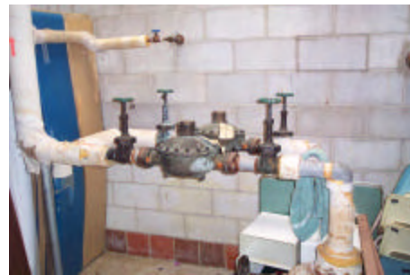
Photo P-2: Water meters.
