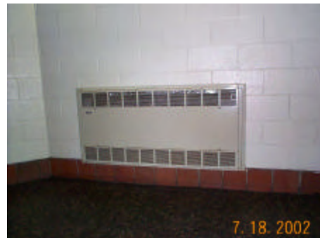
Photo M-2: Cabinet heater in vestibule
