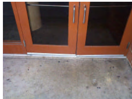
Photo HC-2: Existing Concrete Slab Settlement at Main Entrance Doors
