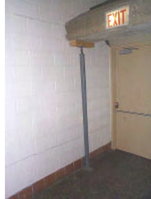
Photo S7: Main Ice Rink – Eastern End of Concrete Grandstand – Shoring adjacent to pinched doorframe.
