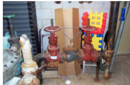
Photo FP-1: Single check backflow preventer on fire protection service.
