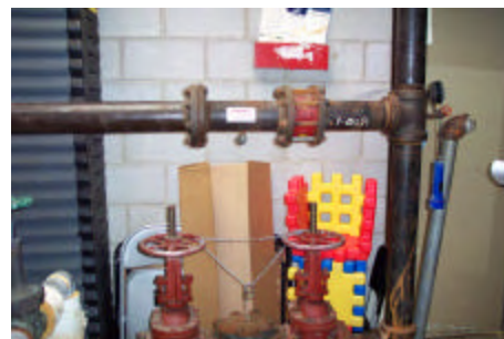
Photo FP-3: Chained and locked valves on fire protection service.
