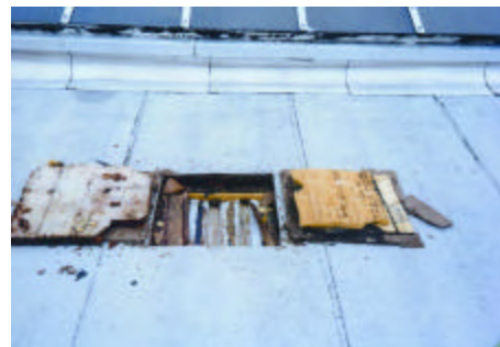
Photo R-5: General view of test cut #2. The main skylight is in the background.
