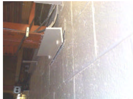
Photo S-2: Main Ice Rink – Joist Bearing - Southern Wall – Roof joist bottom chord connection to masonry wall.
