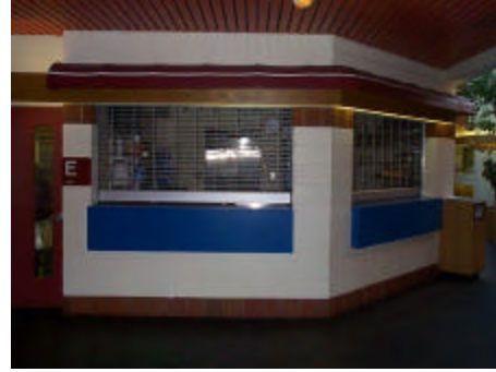
Photo HC-4: Non-compliant Food Service Counter
