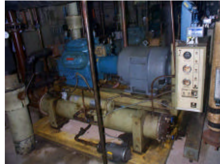
Photo RF-1: Compressors.
