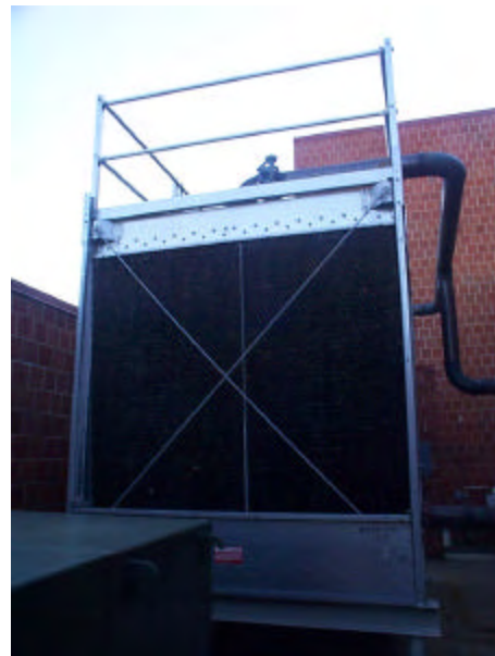
Photo RF-2: Cooling Tower.
