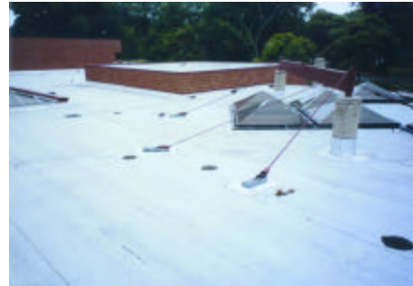
Photo R-1: General view of a portion of the lower roof areas.
