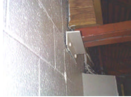
Photo S-1: Main Ice Rink – Joist Bearing – Southern Wall - Roof joist bottom chord connection to masonry wall.
