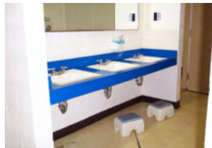
Photo P-3: Plumbing Fixtures.
