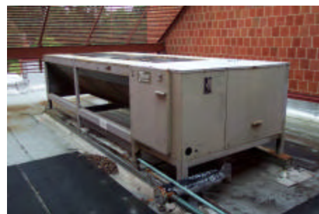
Photo M-3: Roof mounted condensing unit
