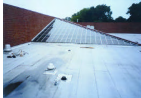
Photo R14: General view of the main skylight. The coping on the diagonal wall was loose.
