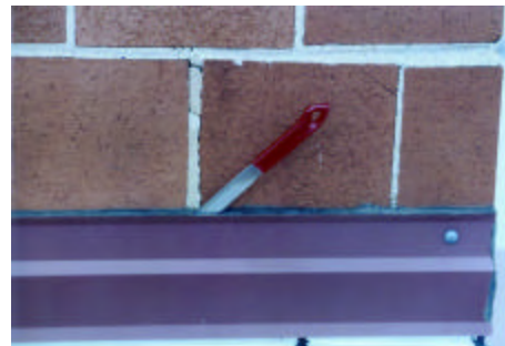
Photo R-12: The putty knife is in an opening where the sealant is no longer bonded. Note the cracked mortar joint.
