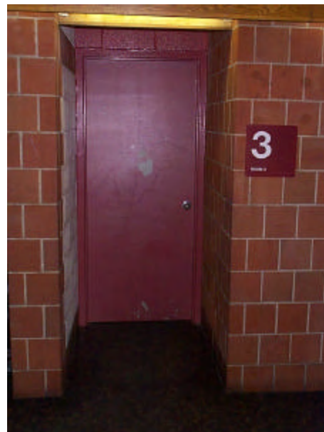
Photo HC-5: Non-compliant Door Into Team Room
