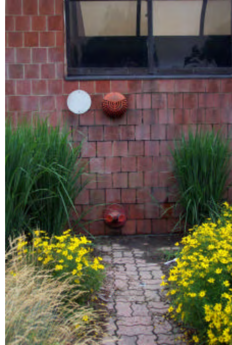
Photo FP-2: Fire department siamese connection and outside electric alarm bell.
