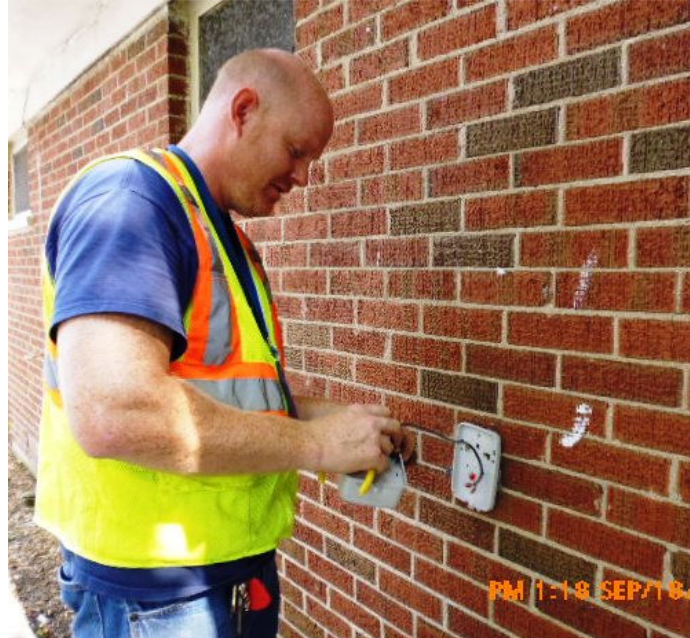
A Utilities Department employee installs a new remote water meter reading unit on the exterior of a home as part of the Advanced Metering Infrastructure (AMI) project. This unit makes it possible for meter readings to be transmitted via wireless network without City staff having to visit each property to manually read the meters.
