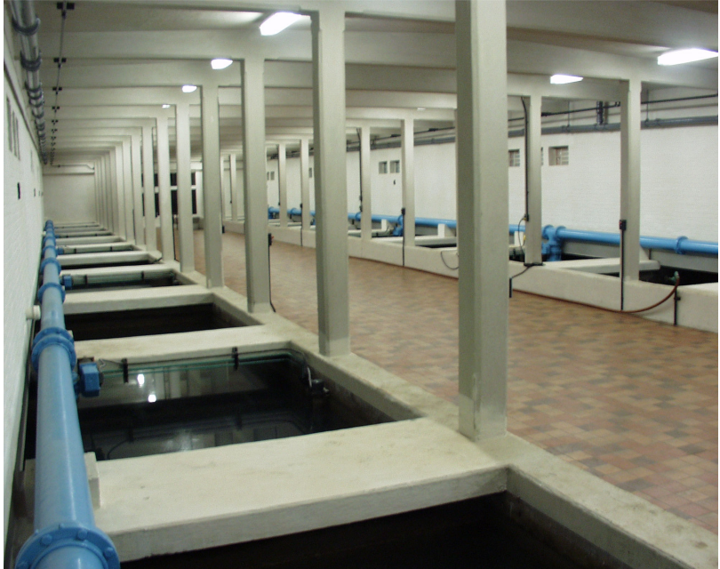
Filters 1 – 12 in operation at the Evanston Water Treatment Plant
