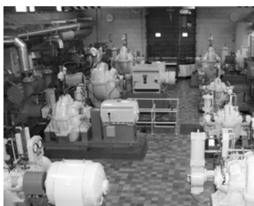
...to our Pumping Facility...
