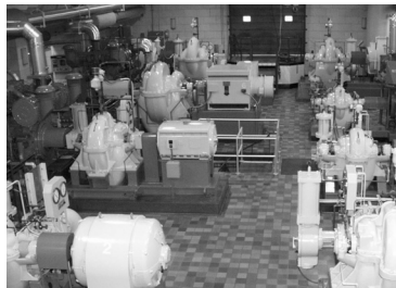
...to our Pumping Facility...
