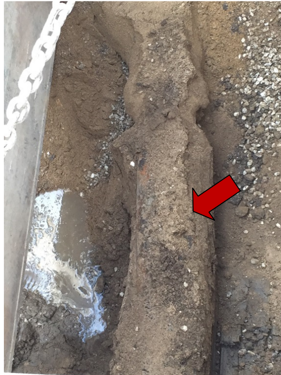
Photo 60: Sample “Exterior Pipe Crust 71+50/7” was collected on 8/20/15 at 9:30 from a depth of 7 feet. Sample is associated with a 10-inch diameter, N-S, water main down center of Dodge (now abandoned). Sample consists of crust scraped from the main (see red arrow). Photo shows encrusted pipe laying in angled trench at Mulford and Dodge. Photo facing south. By Kramer.
