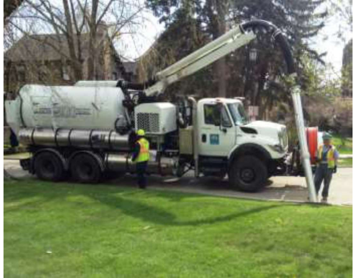
Sewer Division staff operate a sewer cleaning truck to remove debris from a catch basin.
