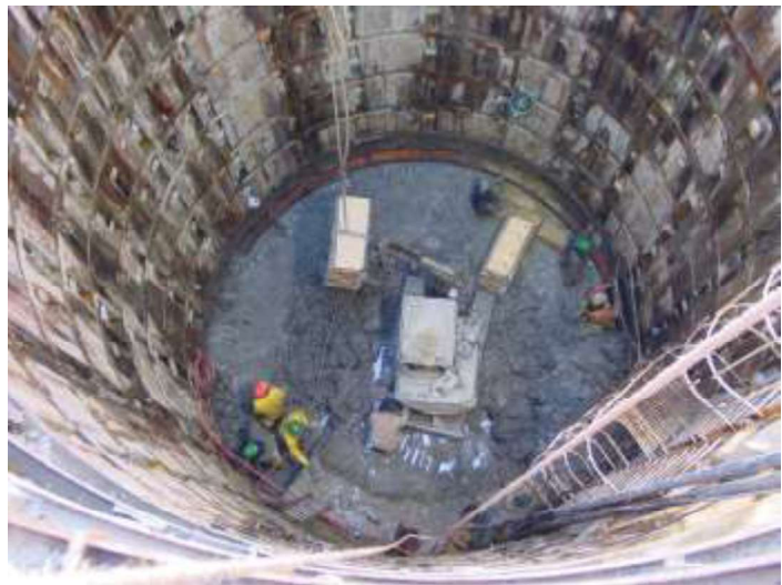
This drop shaft was one of the starting points for a tunneling machine that installed Evanston's relief sewers as a part of the Long Range Sewer Program in 1992 – 2008. Relief sewers are installed at depths of up to 60 feet to efficiently collect and transport large volumes of stormwater without impacting customers and other utilities.
