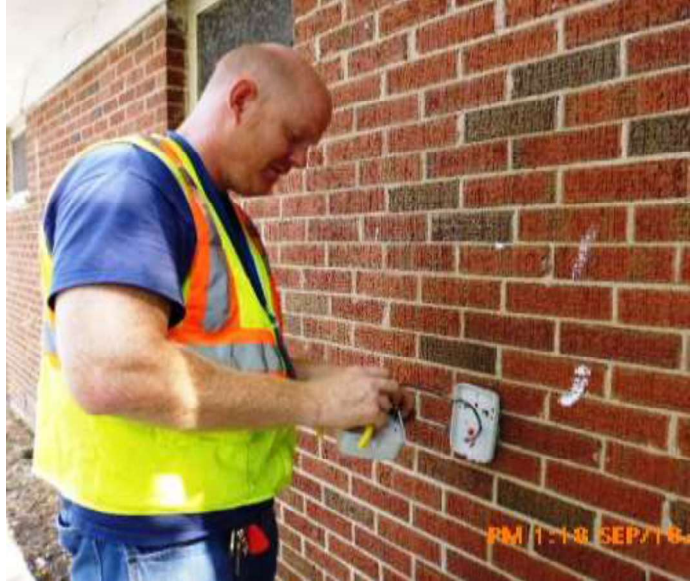
A Public Works Agency employee installs a new remote water meter reading unit on the exterior of a home as part of the Advanced Metering Infrastructure (AMI) project. This unit makes it possible for meter readings to be transmitted via wireless network without City staff having to visit each property to manually read the meters.
