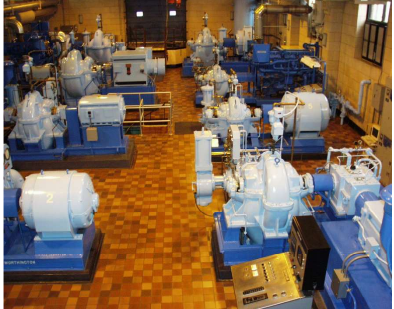
High Lift Pumping Station at the Evanston Water Treatment Plant
