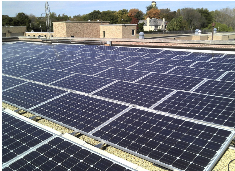
25 kW Array of Solar Panels on Evanston's High Lift Pump Station Roof
